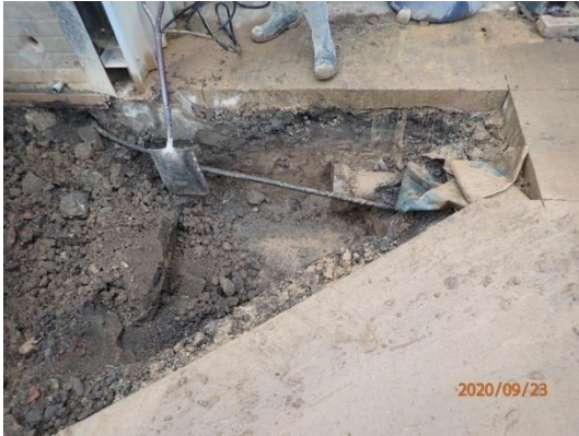
Plate 31: Hand excavations around the area of a modern drain, from the north
