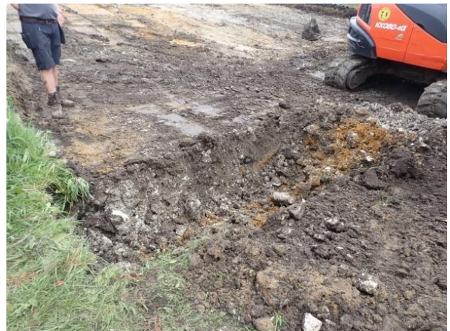
Plate 53: Excavation of the trench at the southern end of the site, from the south-west
