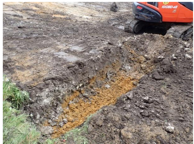
Plate 54: Excavation of the trench at the southern end of the site, from the south-west
