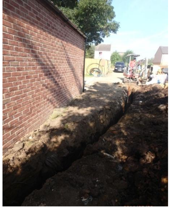
Plate 26: Excavation of the second service trench, from the east showing the location of Representative Section 5
