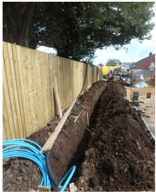
Plate 13: Excavation of the first service trench, from the south showing the location of Representative Section 1
