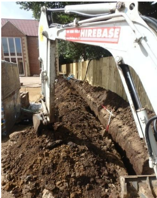
Plate 15: Excavation of the first service trench, from the south showing the location of Representative Section 3
