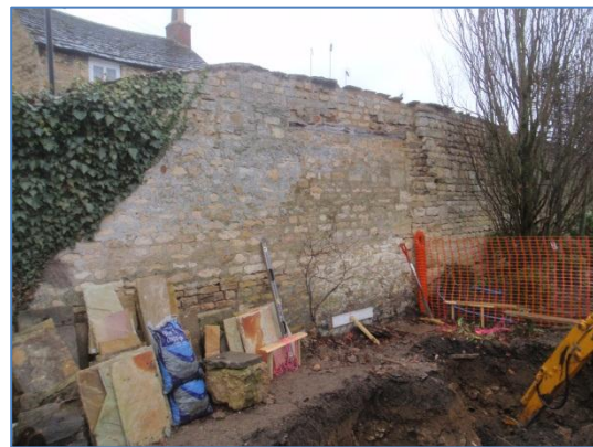
Plate 8: Infilled window opening with timber lintel in the western site boundary wall, from the east
