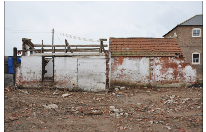
40. Northeast elevation of Building F (left) with later Building H (right and centre), looking SW
