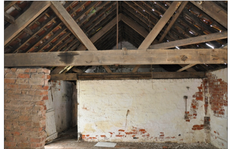
20. Former southeast gable of Building C, later adapted as an internal wall following extension by Building E, looking SE
