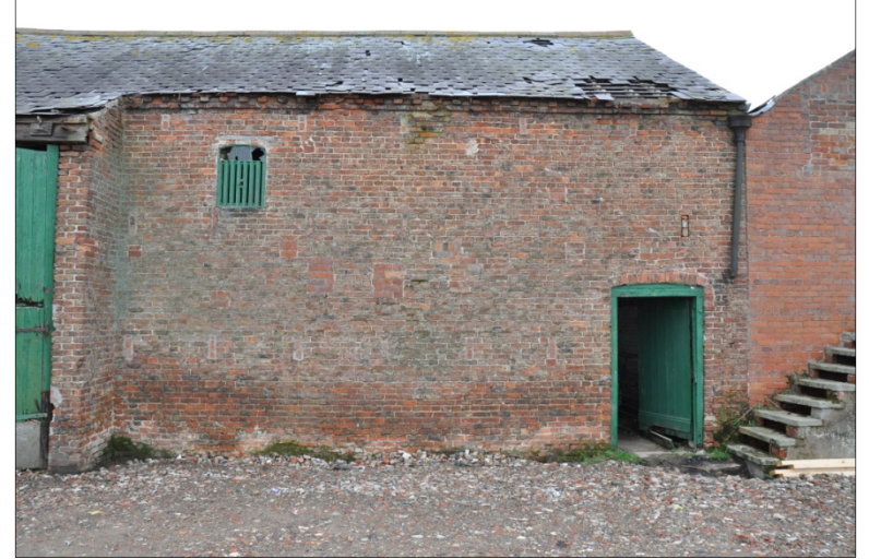
7. Detail of Building A looking SW, showing traces of former perpendicular building at this location
