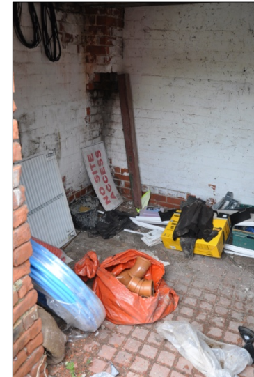
51. Interior of the boiler house showing base of chimney (centre top), looking W
