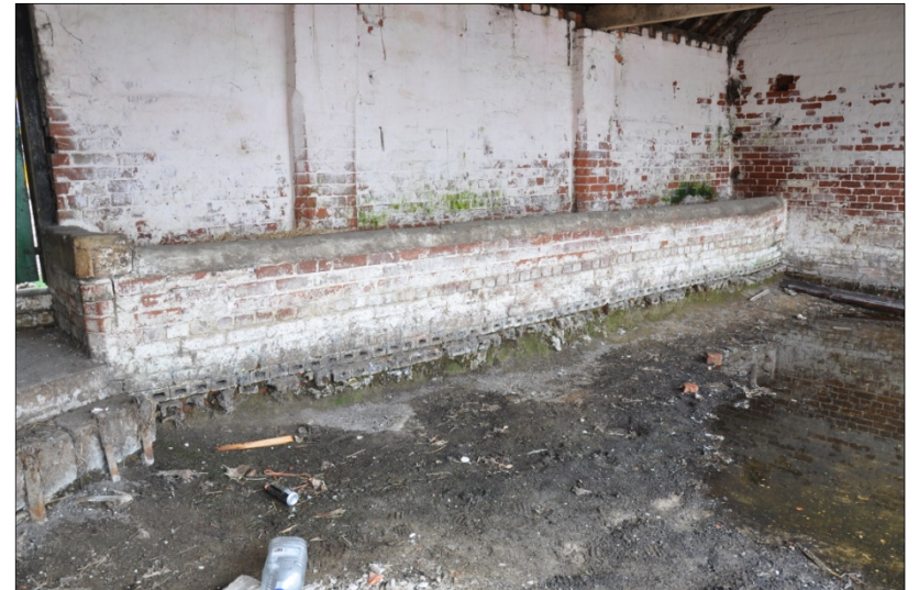
36. Built-in feeder in covered stockyard, looking N
