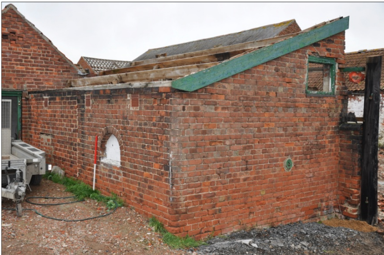
39. Southeast and southwest elevations of Building F showing lunette-shaped hatch (later blocked) for feeding kitchen waste, looking N
