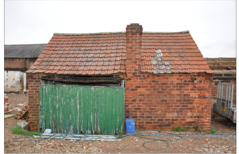
47. Southwest elevation of Building H showing sty (left) and boiler house with small chimney (right) for boiling pigswill, looking NE
