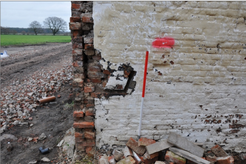
15. Detail of southwest elevation of Building B showing socket of built-in feeder in demolished building, looking NE
