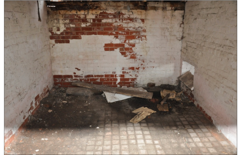
49. Interior of northwest bay of Building H showing pigsty with feeding chute (right), looking NE
