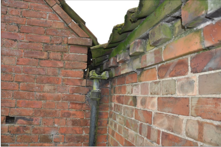
41. Inelegant junction of Building G and Building E, requiring use of a V-gutter, looking S
