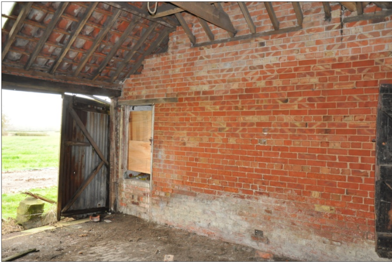
37. Interior of northeastern bay of Building E (possible cake store?), looking S
