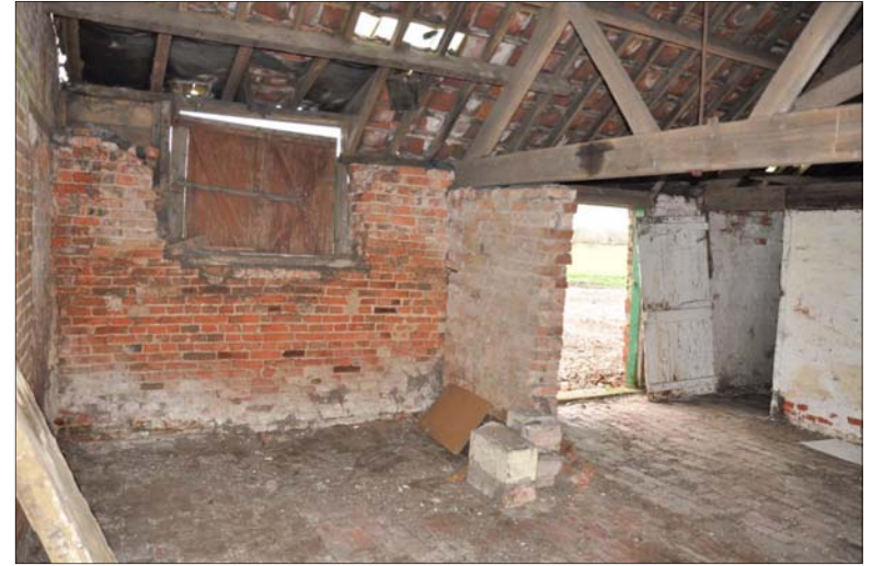
22. Interior of Building C showing later window and internal wall, looking E
