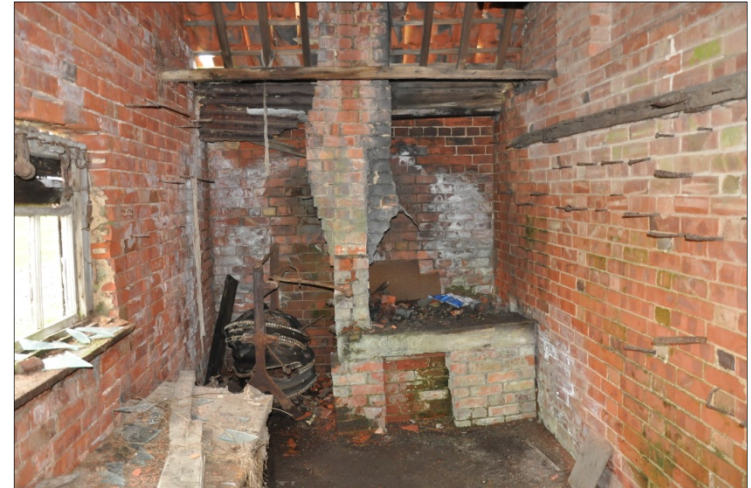
44. Interior of forge in Building G showing forge, hand bellows, tool hooks on wall (right) and work bench (left), looking SW
