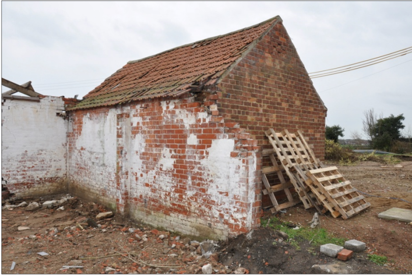
48. Northeast and northwest elevations of Building H showing yard wall with gateway (right), looking S
