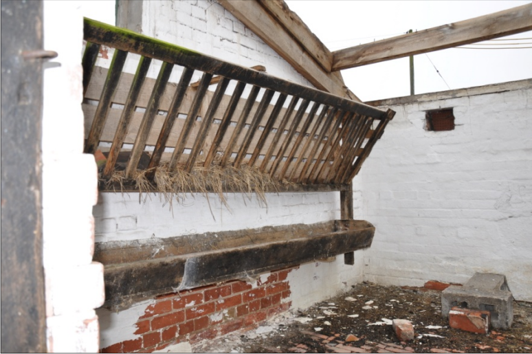
46. Detail of original pigsty (building F), later extended (Building H) and converted to a loose box, looking S
