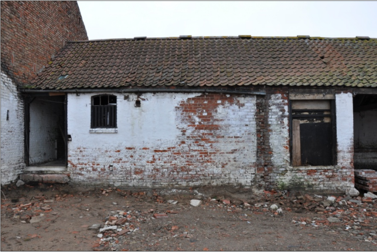
21. Southwest elevation of Building C (left and centre) with building break to Building E (right), looking NE
