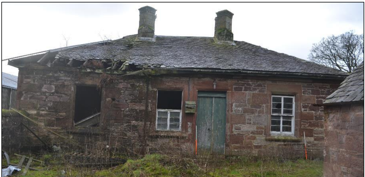
Plate 5: A number of the structures noted were in a poor state of repair (SBR Photograph 013)
