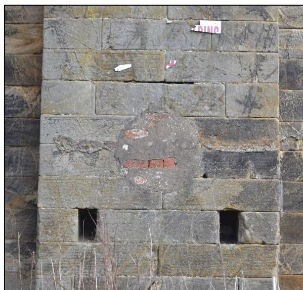
Plate 12: Detailed view of the blocked steam hole. Note the raggle running across the opening (Photograph 038)
