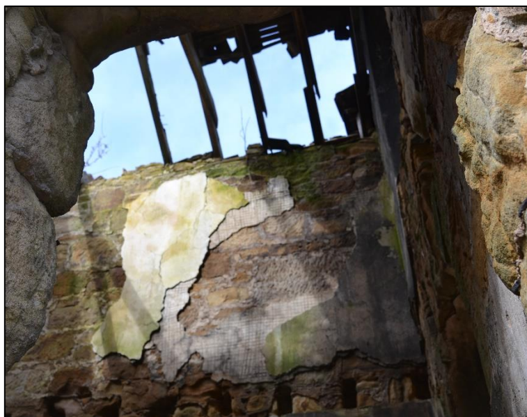
Plate 3: View of the interior showing the poor condition of the roof (Photograph 024)
