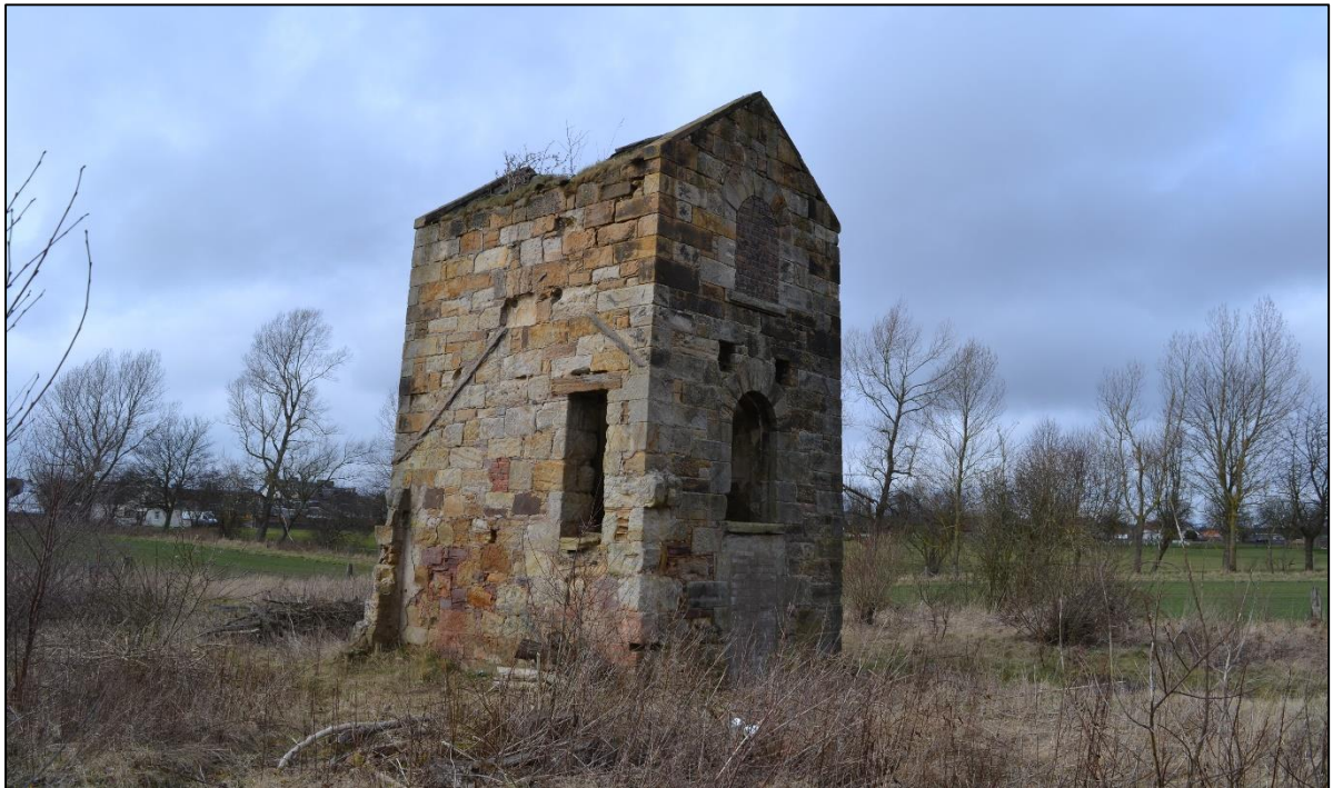
Plate 2: The Beam Engine House from the north west. Note the indications on the fabric of the building showing the presence of now demolished structures (Photograph 007)
