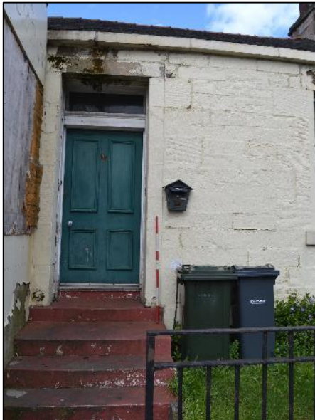
Plate 14: Main entrance in external façade (South facing) fronting onto St John's Road (Photograph 037)
