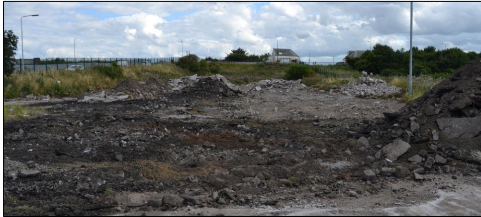
Plate 3: Looking SE across site following removal of the tarmac and concrete (Photograph 034)
