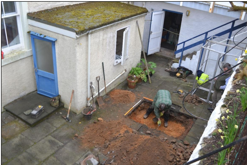
Plate 5: Looking across the courtyard from the north east. Note the drop from the top of the retaining wall, indicating significant landscaping (Photograph 012)
