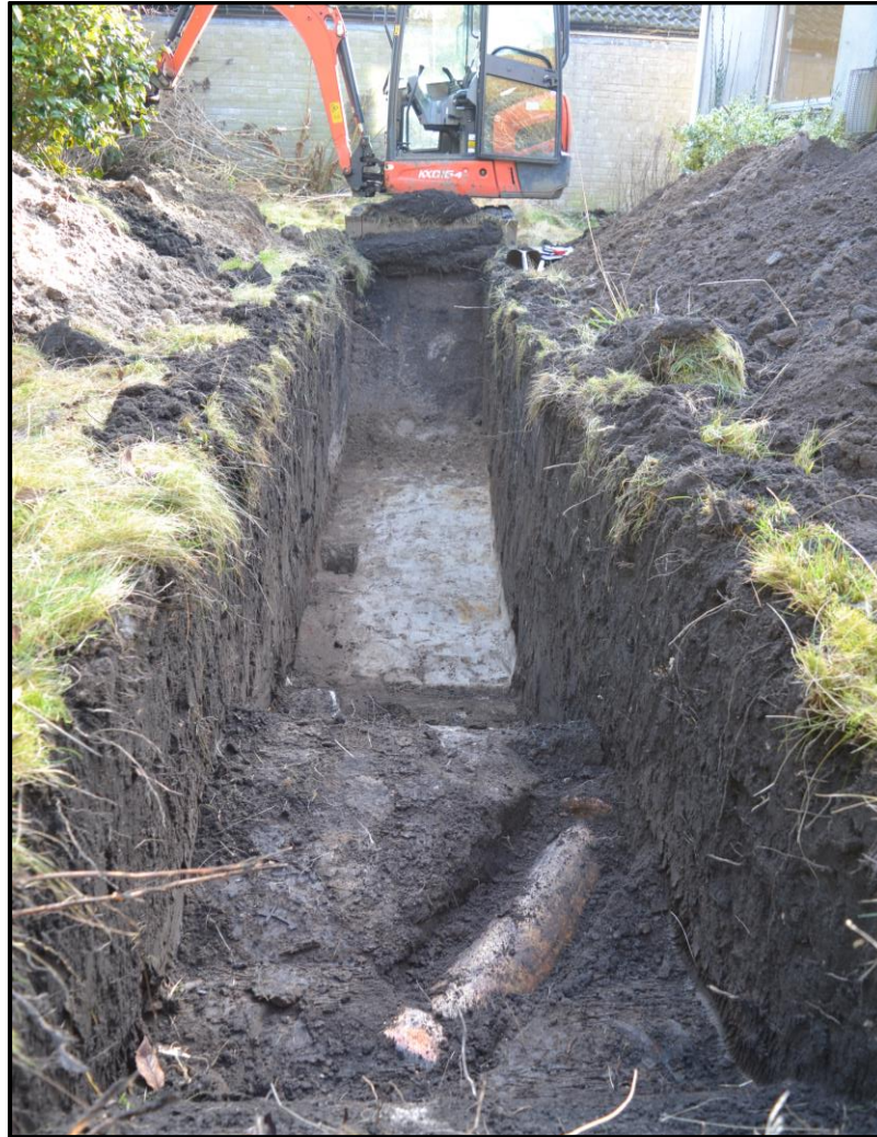
Plate 1: Working shot showing Trench 1 being opened. Large earthenware pipe visible in foreground
