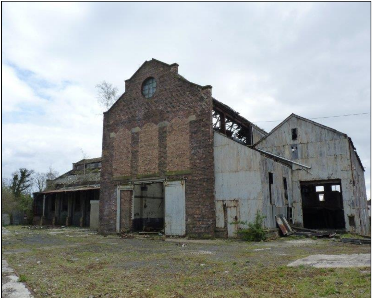
Plate 2: North elevation showing the demolished area of the corrugated steel sheet extension (right) and the building element to the east (left side) ( https://www.buildingsatrisk.org.uk/search/keyword/Victoria%20road/event_id/892403/building_name/victoria-power-station-victoria-road-kirkcaldy 19/08/18)
