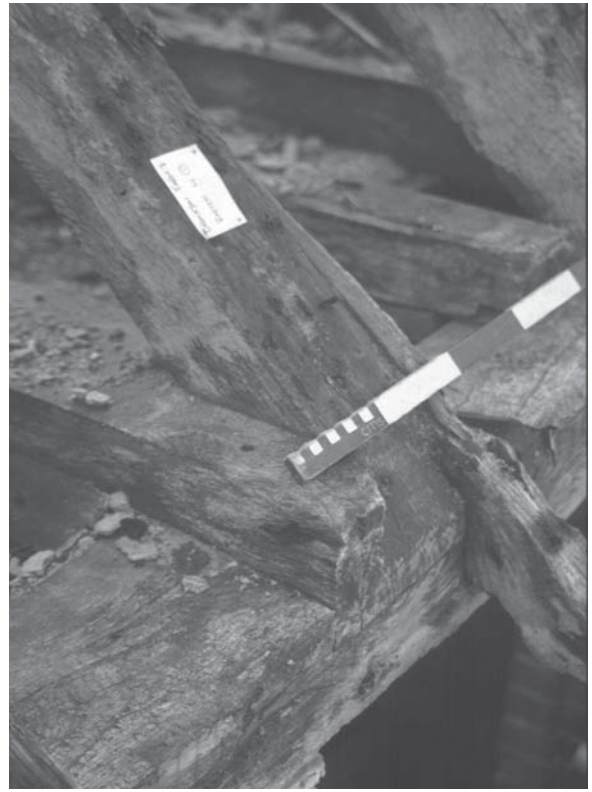
(b) tie beam sawn off flush with outer face of wall plate
