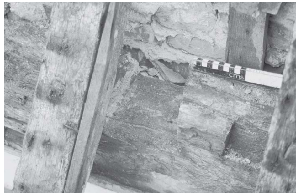
(b) Redundant, former tie dovetail in eastern wall plate
