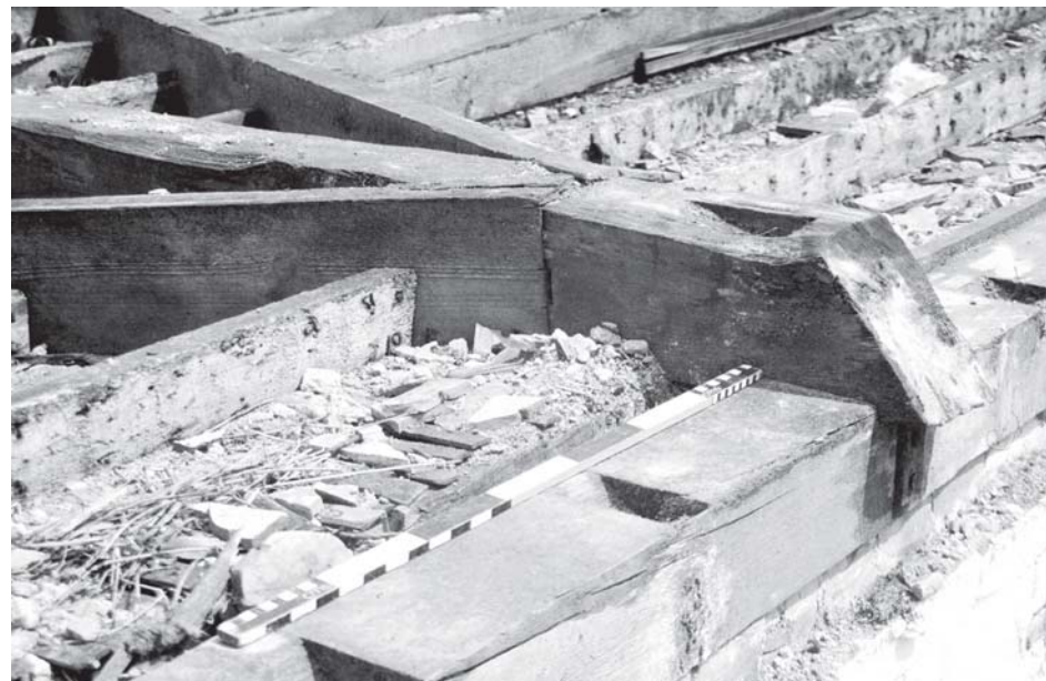
(b) Detail of jointing of tie at south plate; note iron strapping reinforcement
