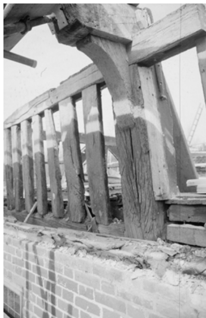
Plate 1: Phase I close studwork of upper hall wall, bay III (note transverse bracket. CF2).
