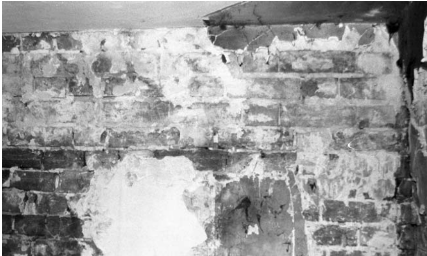
Figure 24: Room GF02 detail of rebuild of upper 4-5 courses of brickwork in west wall
