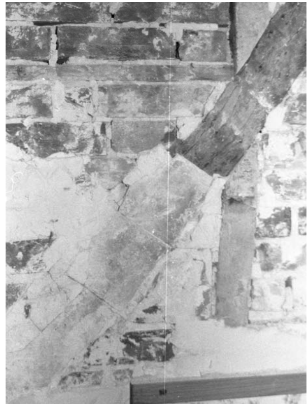
Figure 18: Room GF02, north wall: detail of peg tiles used to level up wall surface prior to plastering
