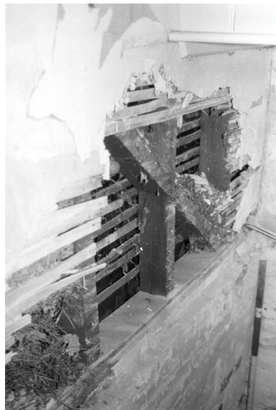
Figure 15: Room GF06, upper storey studwork resting brickwork of Ground floor within stairwell
