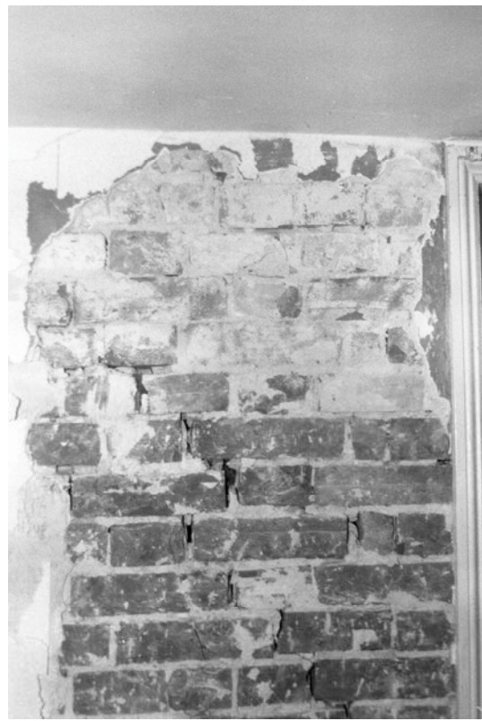
Figure 22: Room GF03: detail of rebuild of upper wall to south of west window
