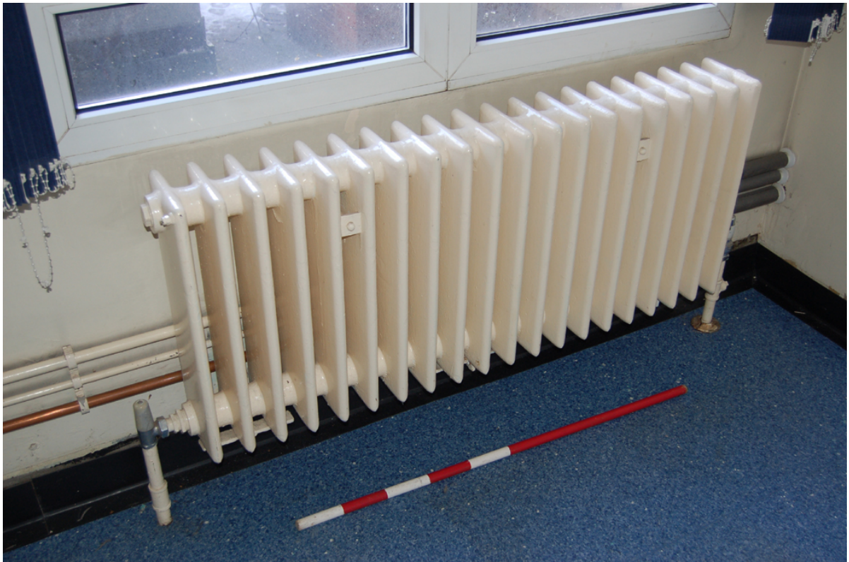
Plate 27: Primary 20 column radiator.
