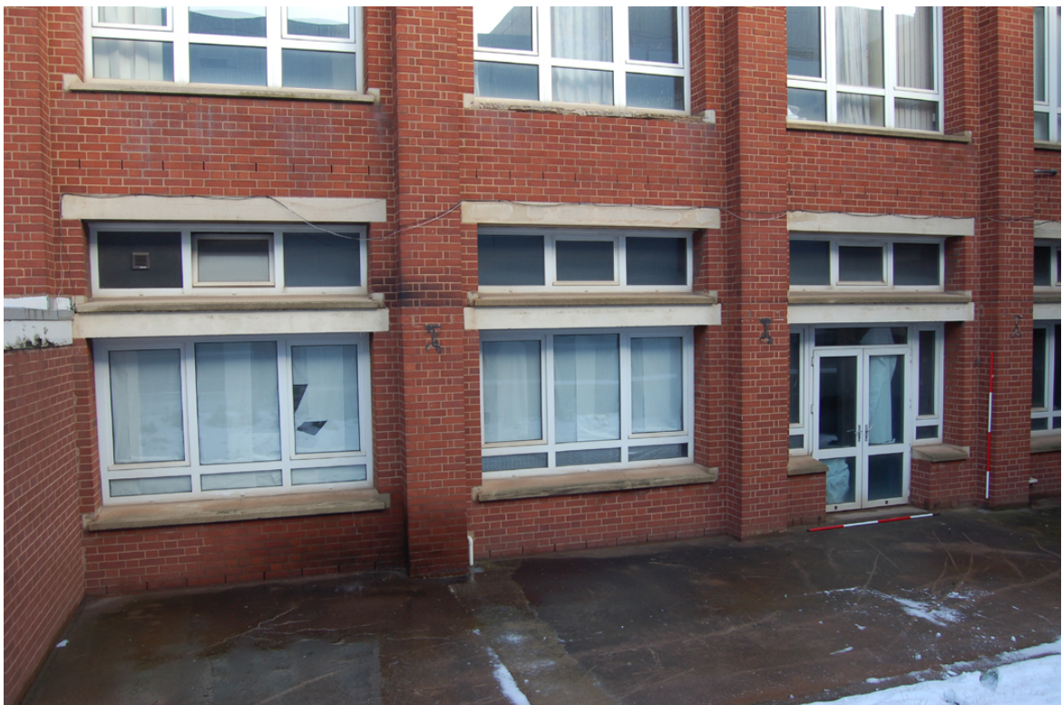
Plate 14: Wider fenestration of south elevation, NB: split GF windows indicating level of former canopy, originally supported by projecting RSJs within brickwork piers.
