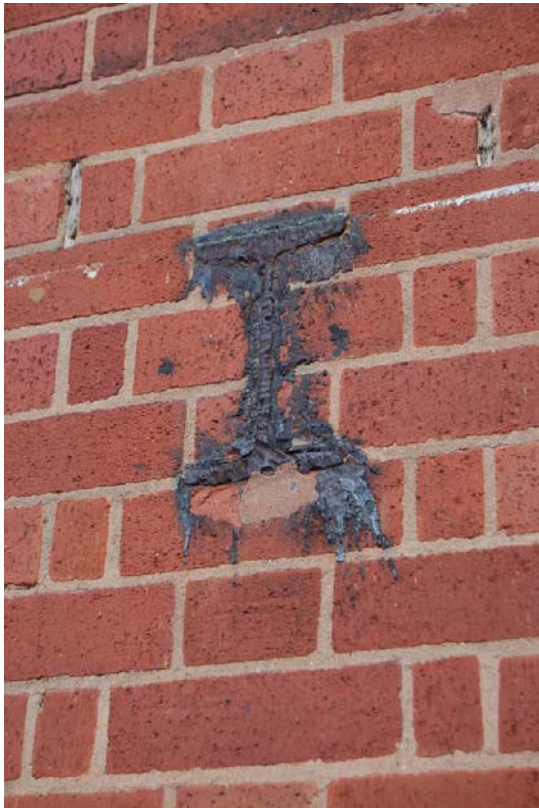
Plate 15: Detail of sawn off RSJ in brickwork pier of south elevation, formerly supporting canopy.
