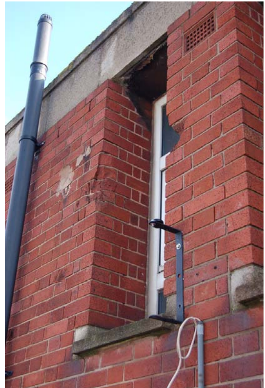
Plate 19: Shrapnel damage in west elev.
