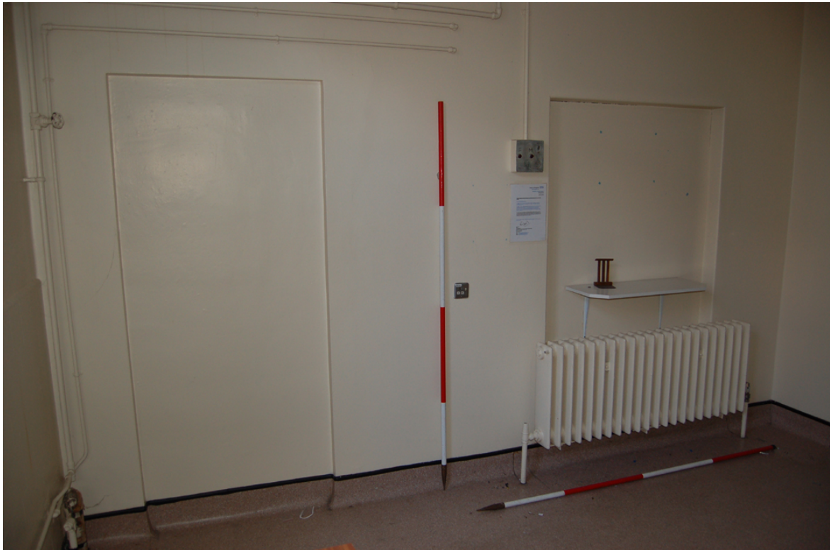
Plate 38: Blocked door and window openings within west wall of [1F06;] (former duty room).
