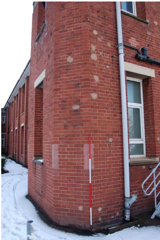
Plate 18: Shrapnel damage at NW corner.
