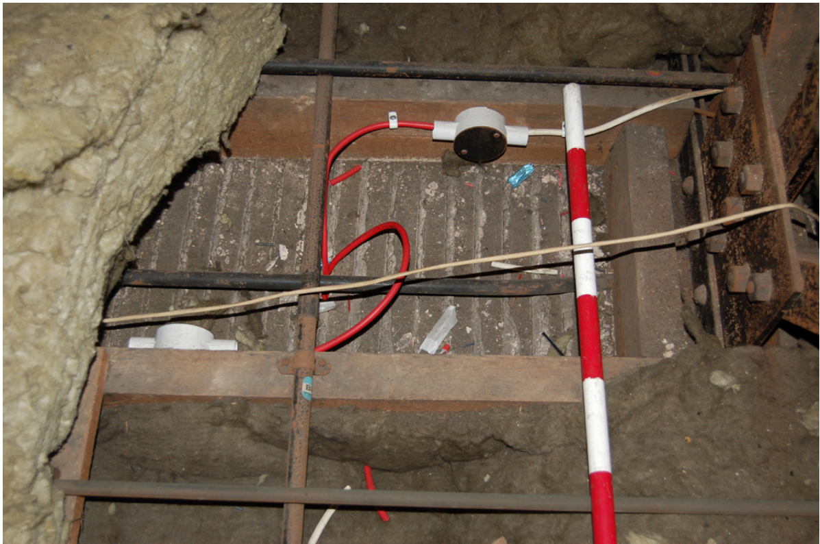
Plate 52: Original lath and plaster ceiling of first floor level visible within roofspace.
