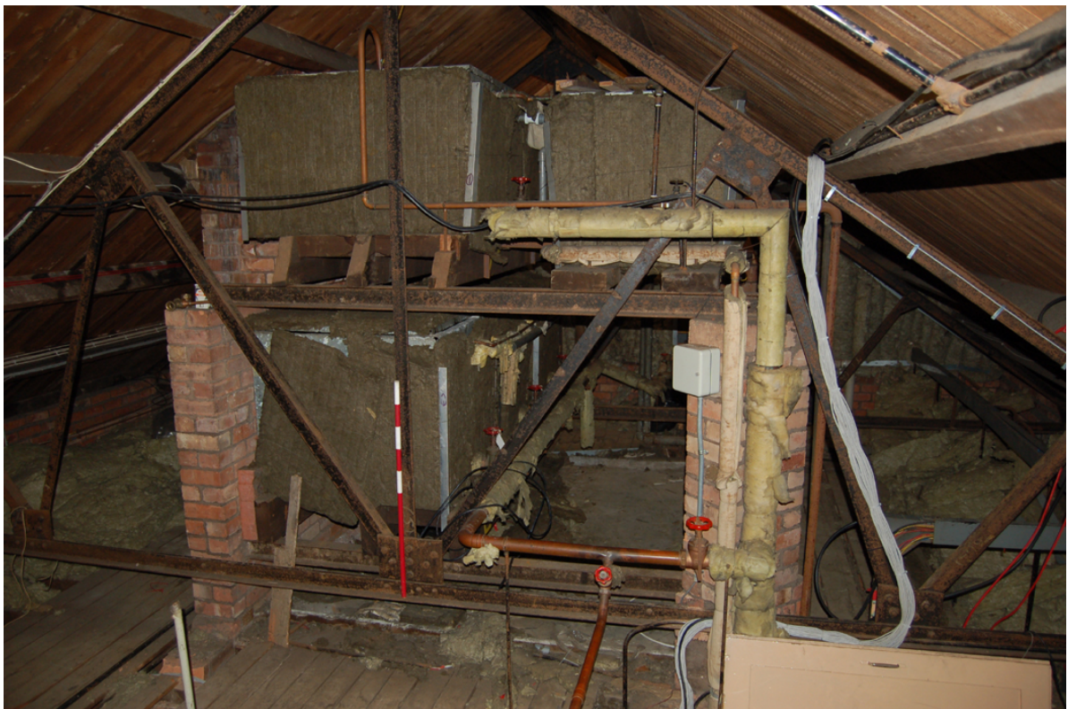
Plate 51: Lowered ceiling level and water storage tanks over central 'core' area of block.
