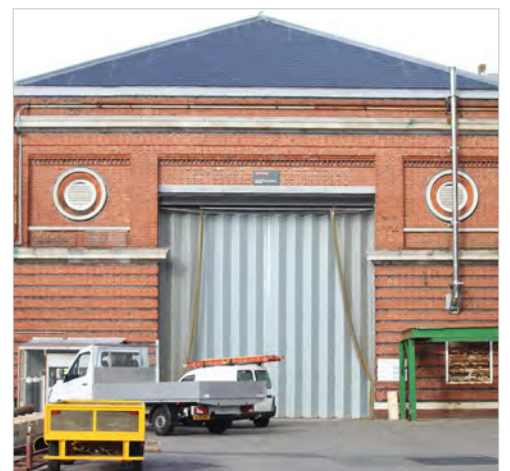
Fig. 59. South elevation of Portsmouth Gunnery Mounting Store (1896, 2/165) with nets to keep out birds in the summer. A. Coats 2013. Reproduced with the permission of the MoD.
