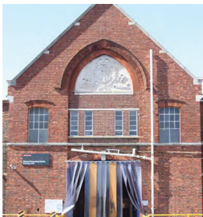
Fig. 58. Original bay and entrance of Portsmouth Torpedo Workshop (1886, 3/69), with plastic strips to keep out birds in summer. A. Coats 2015. Reproduced with the permission of the MoD.
