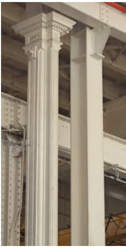
Fig. 52. Neoclassical iron columns cast in an industrial style inside Portsmouth Main Pumping Station No. 1 (1878, 2/201). A. Coats 2015. Reproduced with the permission of the MoD.
