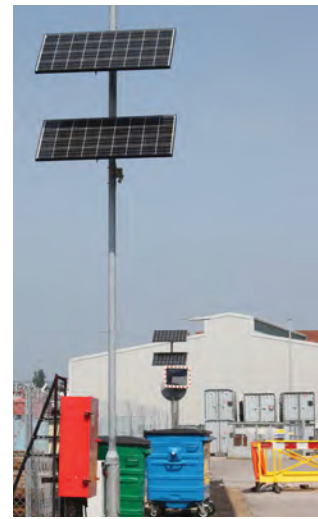
Fig. 42. Panel of photovoltaic cells to generate electricity at Portsmouth in 2013, south of the Lub Oil Store (3/251). A. Coats 2013. Reproduced with the permission of the MoD.
