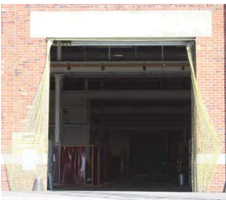
Fig. 57. Modified south entrance to Portsmouth Armour Plate Shop/No. 1 Ship Building Shop/Multi-functional Workshop (1867, 2/172) supplied with nets to keep out birds in the summer. A. Coats 2015. Reproduced with the permission of the MoD.
