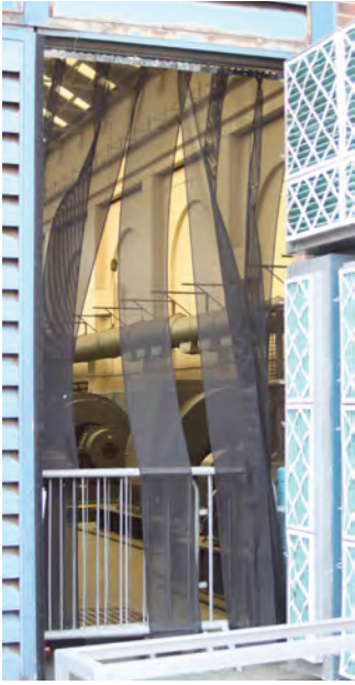
Fig. 60. Portsmouth Central Boiler House plastic door strips to keep out birds in summer (1907, 2/19). A. Coats 2013. Reproduced with the permission of the MoD.
