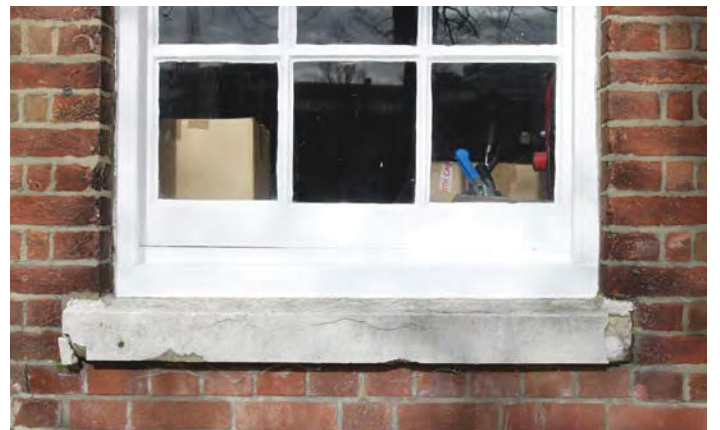
Fig. 39. Concrete sill showing deterioration, Portsmouth Storehouse No. 34 (c.1786, 1/149), modified after Second World War bomb damage. A. Coats 2013. Reproduced with the permission of the MoD.
