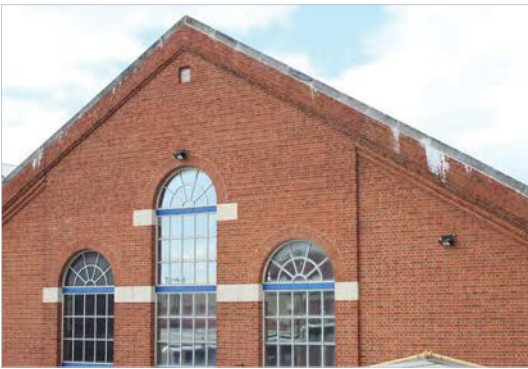
Fig. 54. East elevation showing the 1994 brick gable pediment to the extension of Bay 1 of Portsmouth Factory/100 Store (1903, 3/82), designed to appear similar to the original gable pediments. A. Coats 2013. Reproduced with the permission of the MoD.
