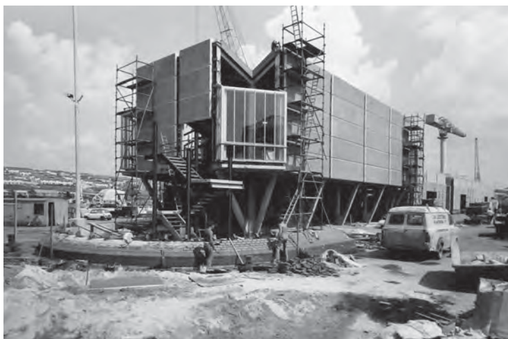
Fig. 124. NAAFI building (July 1977). TNA, CM 20/80 (1976). PSA: Devonport: Works Projects. Photograph albums. Fleet Maintenance Base Devonport: book no. 4. Reproduced with the permission of The National Archives.
