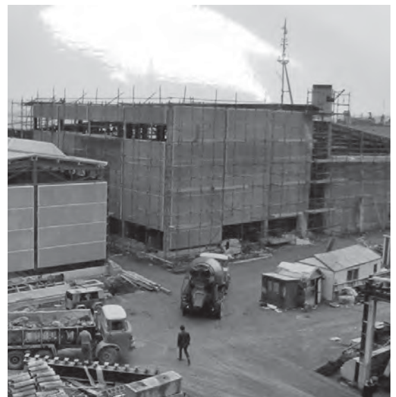
Right: Fig. 167. Submarine Refit Complex, N018 (November 1975). TNA, CM 20/78 (1975). PSA: Devonport: Works Projects. Photograph albums. Fleet Maintenance Base Devonport: Foundations book no. 2. Reproduced with the permission of The National Archives.
