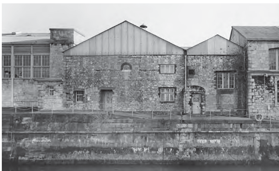
Fig. 70. BB96/03891. Devonport South Yard South Smithery (S126) photograph of north elevation of centre building (29 Feb 1996). ©Crown copyright.HE.
