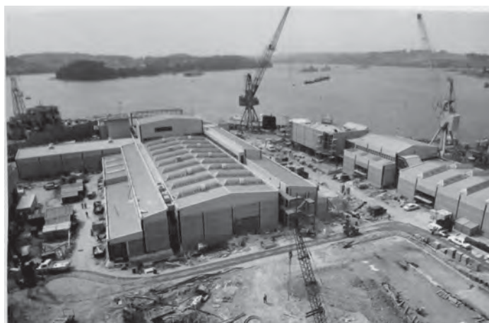
Fig. 126. NAAFI building (July 1977). TNA, CM 20/80 (1976). PSA: Devonport: Works Projects. Photograph albums. Fleet Maintenance Base Devonport: book no. 4. Reproduced with the permission of The National Archives.
