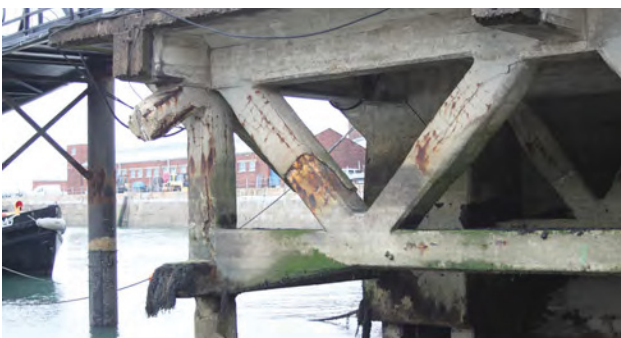
Fig. 231. Southern extent of the concrete and steel trusses forming the undercroft of Portsmouth Boathouse No. 4 (1940, 1/6) on its west (harbour) elevation. A. Coats 2015. Reproduced with the kind permission of Portsmouth Naval Base Property Trust.
