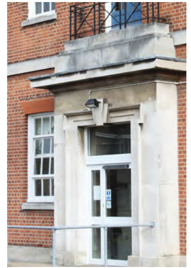
Fig. 278. Entrance to Sunny Walk Offices (1950, 1/31). A. Coats 2013. Reproduced with the permission of the MoD.
