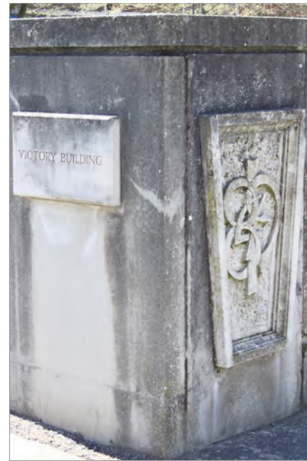
Fig. 347. One of the concrete entrance piers, east of Portsmouth Victory Building (1993, 1/100), dated 1984. A. Coats 2013. Reproduced with the permission of the MoD.
