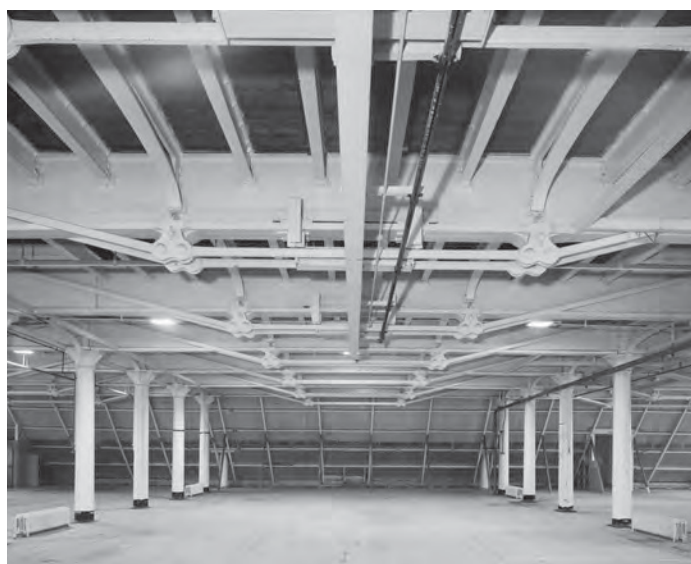
Fig. 262. BB012878. Photograph of the first floor interior of Portsmouth Boathouse No. 6 from the west, before refurbishment in 2001 (11 Jun 1991). ©Crown copyright.HE.
