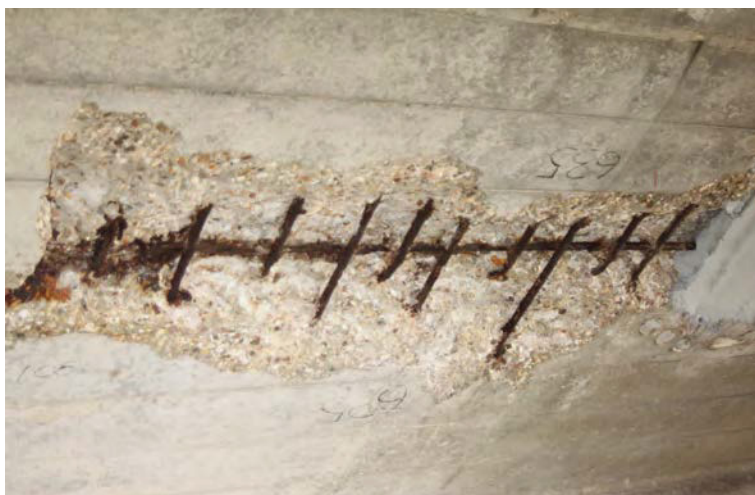
Fig. 238. Underside of Portsmouth Boathouse No. 4 (1940, 1/6) showing the shuttered concrete surface with twentieth century repairs using steel wire which has corroded. Concrete repairs were carried out in 2014–15. A. Coats 2015. Reproduced with the kind permission of Portsmouth Naval Base Property Trust.
