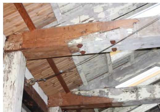
Fig. 375. Interior of the Portsmouth Block Mills (1802, 1/153), showing new roof timber and two beams where traditional scarf joints bond old and new timber. A. Coats 2010. Reproduced with the permission of the MoD.
