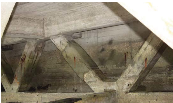
Fig. 233. Northern extent of the concrete and steel trusses forming the undercroft of Portsmouth Boathouse No. 4 (1940, 1/6) on its west (harbour) elevation, showing the shuttered concrete west seawall. A. Coats 2015. Reproduced with the kind permission of Portsmouth Naval Base Property Trust.
