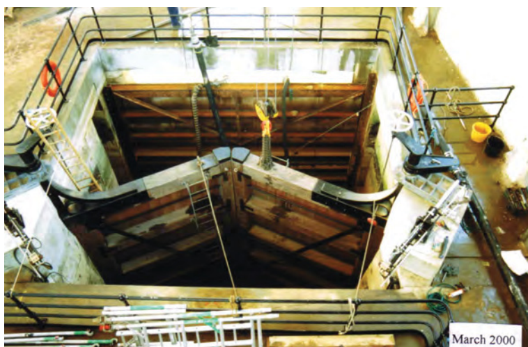
Fig. 249. Photograph of Portsmouth Boathouse No. 4 lock gates: adjustments to gates (PNBPT, 1.3.2000 no. 53). Reproduced with the kind permission of Portsmouth Naval Base Property Trust.
