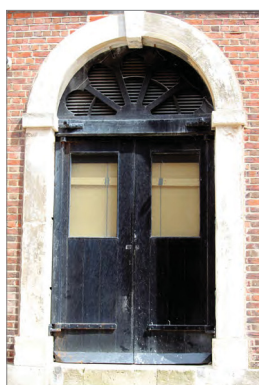
Fig. 315. A rear (west) door of Portsmouth Storehouse No. 10 (1776, 1/59), facing the North Camber. A. Coats 2014. Reproduced by kind permission of the Trustees of the National Museum of the Royal Navy.
