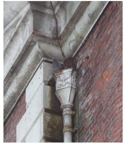
Fig. 378. Portsmouth Steam Factory (1847, 1/208), rainwater hopper, east elevation, dated 1847. A. Coats 2013. Reproduced with the permission of the MoD.
