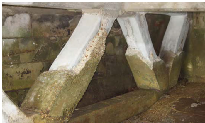
Fig. 234. Northern extent (east end) of the concrete and steel trusses forming the undercroft of Portsmouth Boathouse No. 4 (1940, 1/6) showing the eighteenth century Portland stone north seawall and slipway stones. Concrete repairs to the trusses were carried out in 2014–15. A. Coats 2015. Reproduced with the kind permission of Portsmouth Naval Base Property Trust.
