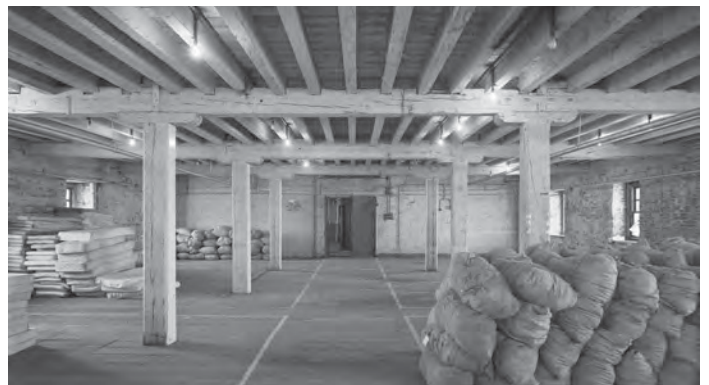
Fig. 308. J186/05/71. Photograph of Storehouse Nos 9, 10 or 11 (28 Apr 1971). ©Crown copyright.HE. It is hoped that the particular storehouse can be identified.
