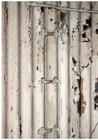
Fig. 327. Original corrugated iron and fittings inside Portsmouth Fire Station (1843, 1/77). A. Coats 2012. Reproduced with the permission of the MoD.
