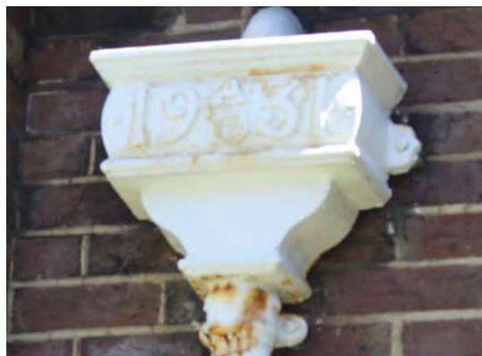
Fig. 331. Rainwater hopper dated 1931 on Portsmouth South Office Block Annexe (1931, 1/87C). A. Coats 2013. Reproduced with the permission of the MoD.
