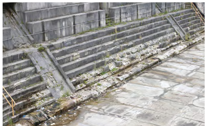
Fig. 339. Portsmouth Dock No. 6 (1700), showing disintegration of the lower altar stones through weathering. Following the straightening of the western jetties for the new Queen Elizabeth class aircraft carriers in the early 2000s, it is no longer connected to the harbour and no longer has the environmental protection of seawater. A. Coats 2012. Reproduced with the permission of the MoD.
