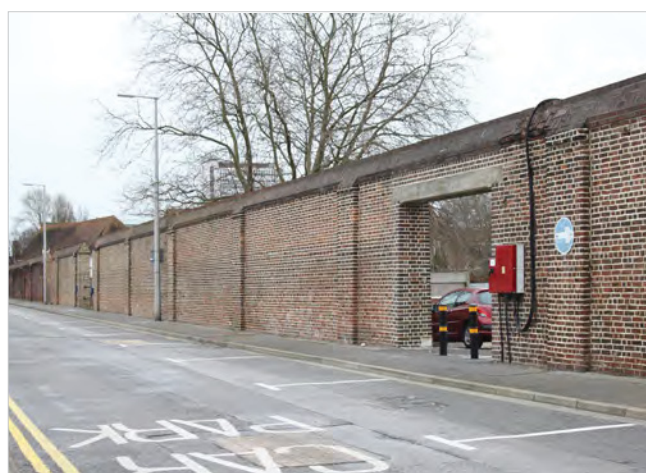
Fig. 209. Original 1711 Portsmouth Dockyard Wall, this section now within the Naval Base between the new and original Marlborough Gates, taken inside the yard as the Marlborough Salient in 1944. A. Coats 2013. Reproduced with the permission of the MoD.
