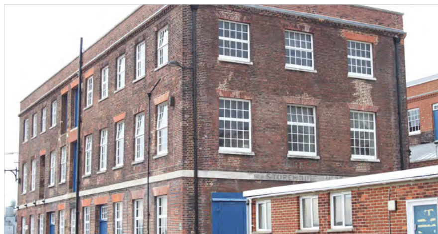
Fig. 374. South elevation of the Portsmouth Block Mills (1802, 1/153), with the external twentieth century fire escapes removed. A. Coats 2010. Reproduced with the permission of the MoD.
