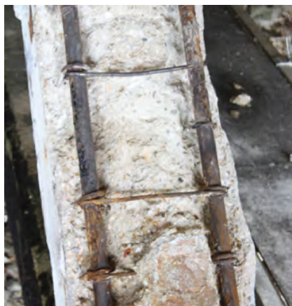
Fig. 236. Underside of a Portsmouth Boathouse No. 4 (1940, 1/6) concrete truss, showing its corroded iron reinforcing bar. A. Coats 2015. Reproduced with the kind permission of Portsmouth Naval Base Property Trust.
