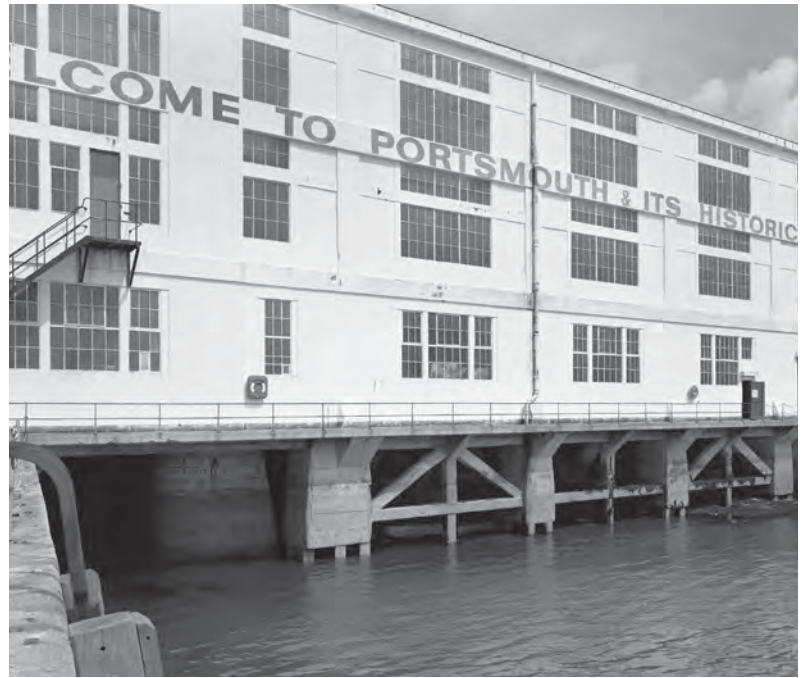
Fig. 229. BB97/09274. West elevation of Boathouse No. 4 showing the concrete supporting trusses at high tide (28 Jul 1997). ©Crown copyright.HE.
