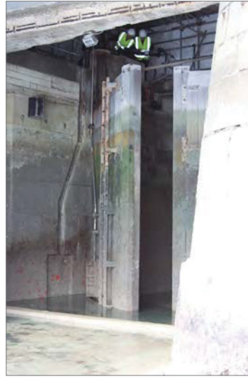
Fig. 240. Lock entrance to Portsmouth Boathouse No. 4 (1940, 1/6), showing the wooden lock gates which connect the channel running beneath Boathouse No. 4 and into the Mast Pond with the harbour. On the right is the battered eighteenth century Portland Stone sea wall, at the top a reinforced concrete beam supporting the building, and on the left shuttered concrete above Portland stone. A. Coats 2015. Reproduced with the kind permission of Portsmouth Naval Base Property Trust.
