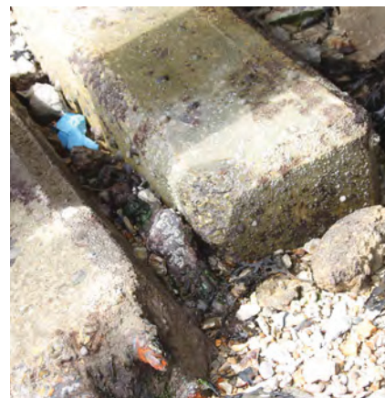
Fig. 237. Unused reinforced concrete beams lying beneath Portsmouth Boathouse No. 4 (1940, 1/6). A. Coats 2015. Reproduced with the kind permission of Portsmouth Naval Base Property Trust.
