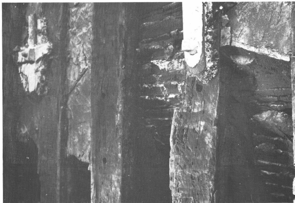
3 (b) The Peacock Inn: Bay 3, first floor, north wall from the interior showing studs and coving brackets, both grooved for infill.
