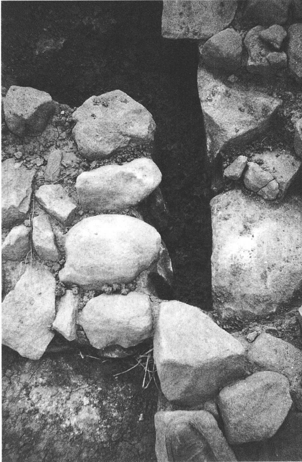
Plate 2: Ockbrook, Little Hay: abutment of internal partition wall to north wall, showing gap inbetween.
