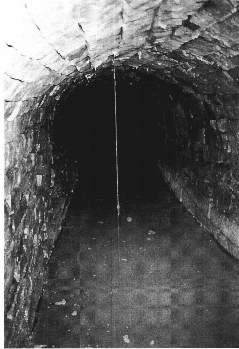
Plate 8: Thornsett Hey coal tunnel in July 2002. It was last used in 1885. (SK 007872).
