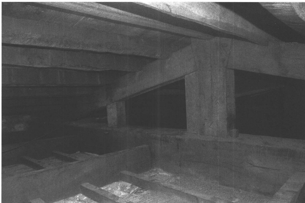
Plate 2: Bolsover Castle: one of shallow trusses of roof of 'Little Castle'; king-post is 0.82m in height.
