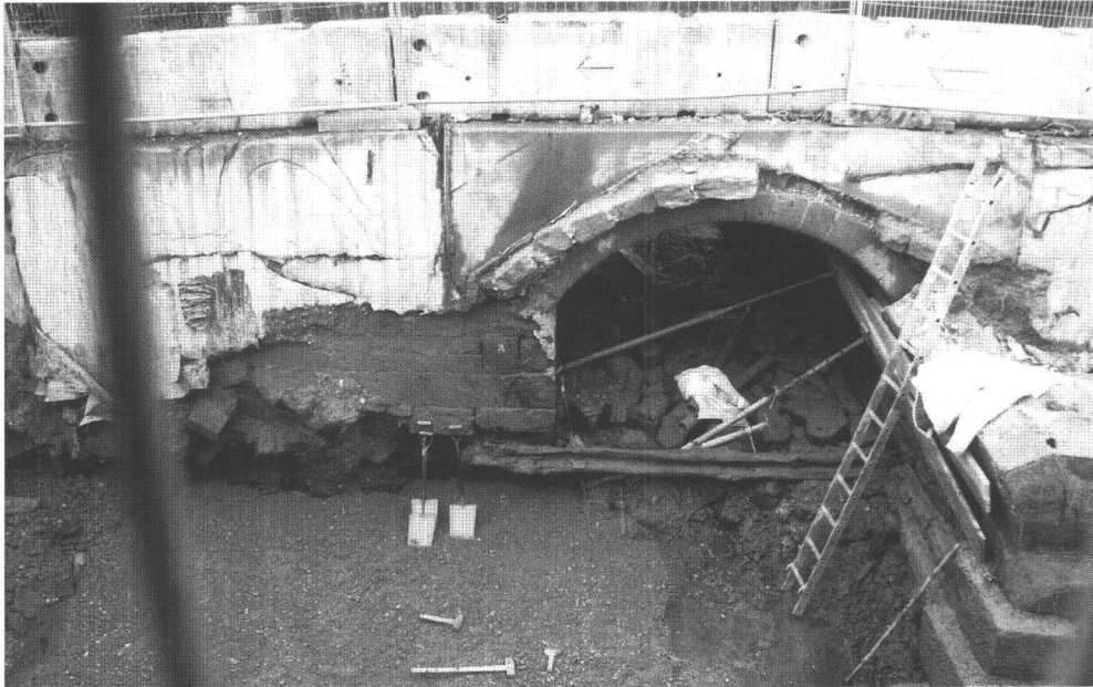
Plate 4: Monk's Flood North Bridge, Egginton: with most of Phase II widening removed before reassembly, west side of Phase I arch revealed together with added stone-collar and, beyond foot of ladder, one of horizontal timbers retaining stone infill; looking south-east; for scale, compare Fig. 1.
