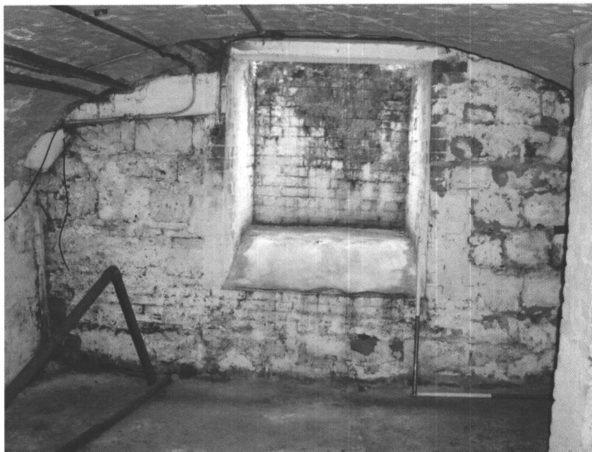
Plate 16: 7a Abbey Lane. Ground floor, south room showing opening in west wall, 2007 (P. J. Steer).
