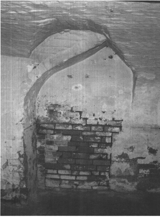
Plate 18: 7a Abbey Lane. Ground floor, south side, partition wall, 2007 (P. J. Steer).
