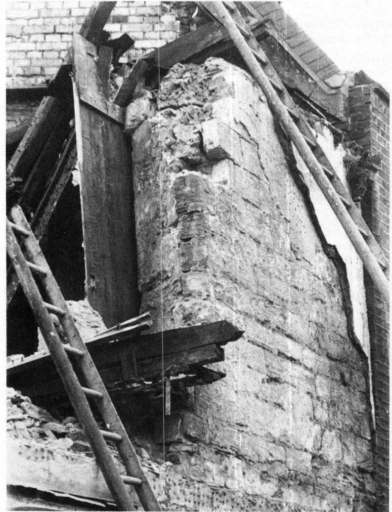
Photo: Colin Shewring Plate XXXIV. The front wall 33 of No.28 partly demolished showing reveal for first floor window.
