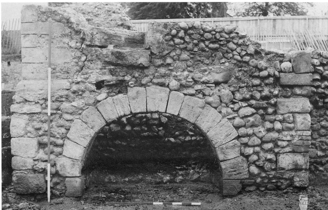
XIX. Arch 1066 in turret 2025, Building 2100. The wall above the arch was rebuilt in the fifteenth century. Vertical scale: 2 metres. Horizontal scale: 1 metre (BWE7)
