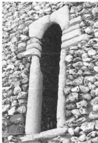
Plate XXII. Pudding Norton, St Margaret: single-splayed window of the second half of the 11th century.
