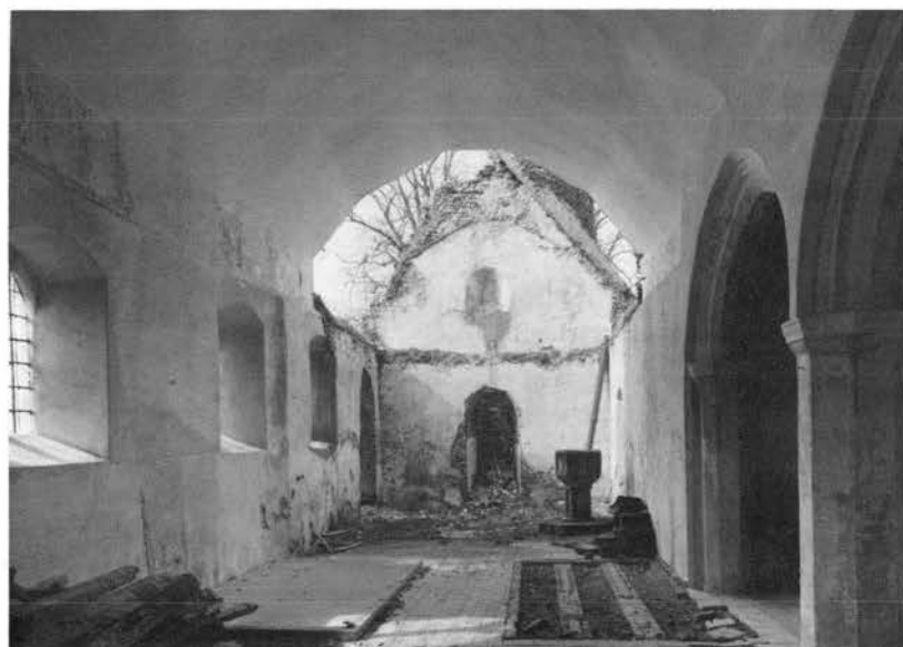
Plate LXII. Morton-on-the-Hill, St Margaret: interior looking west in 1978. The tower collapsed in 1959 destroying part of the nave roof. In the care of the Norfolk Churches Trust since 1979, the west end of the nave has now been sealed off and the rest of the church put in good order. BB79/629 copyright Royal Commission on Historical Monuments (England), 1978.
