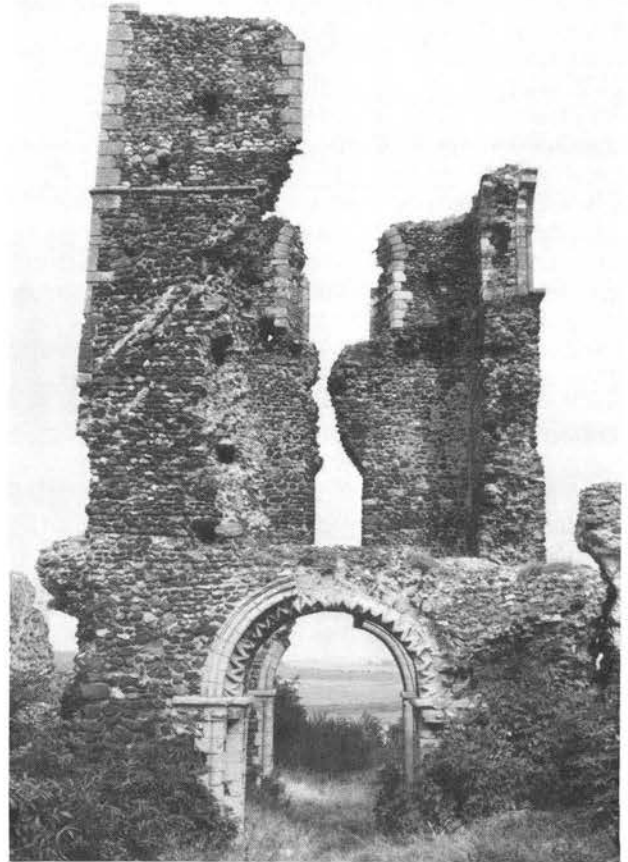
Plate XCII. Bawsey, St James, looking east. The triangular-headed opening above the chancel arch led into the roof-space above the chancel vault.
