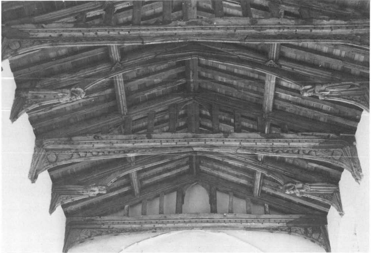
Plate XXXVII. Hockwold, St Peter: magnificent early 16th-century nave roof of arch-braced tie-beams alternating with hammer-beams.
