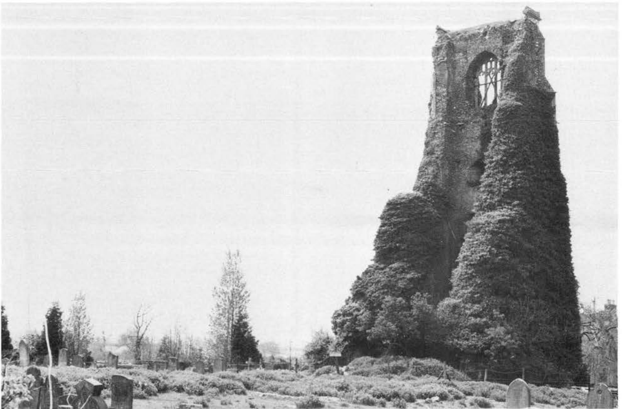
Plate II. Hindolveston, St George: an ill-fated church: the south aisle burned down after being struck by lightning in 1804; then in 1892 half of the tower collapsed and demolished the nave. All photos by the author unless credited otherwise.
