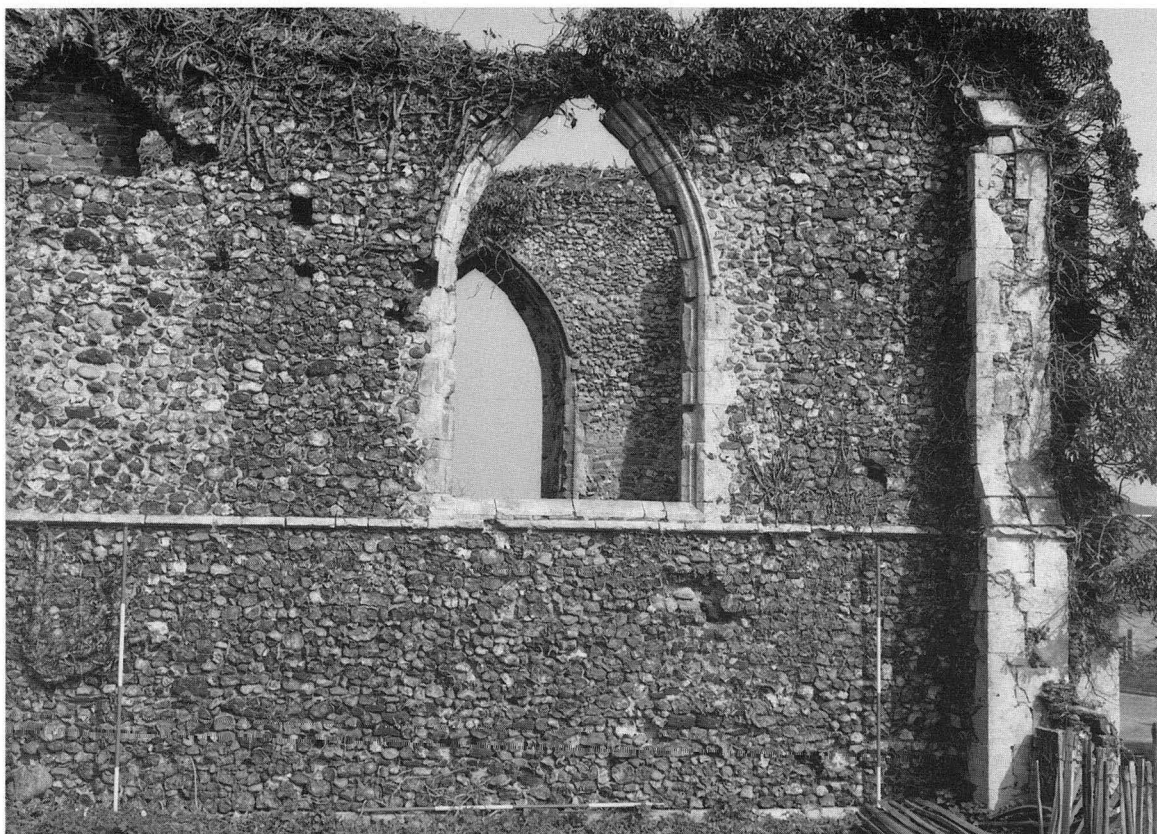
Plate XXX Period II church. Detail of exterior of east end of chancel south wall showing corner buttress, eastern window and blocked central window. (Compare interior elevation, Figure 51). Scales 2 metres. (Photo: B.Lloyd)
