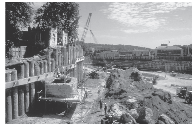
Plate 6.18 Excavation of the well shaft (50108, Period 3.1), viewed from the west after reduction of surrounding area (Area 5)
