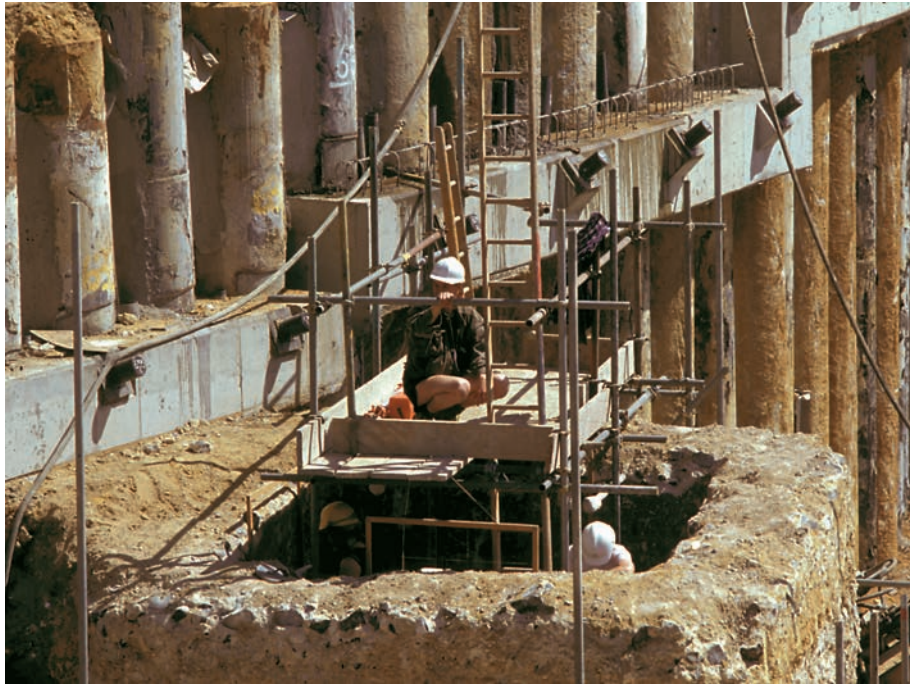
Plate 9.1 Barbican well during excavation of late medieval/transitional fills, following surrounding ground reduction
