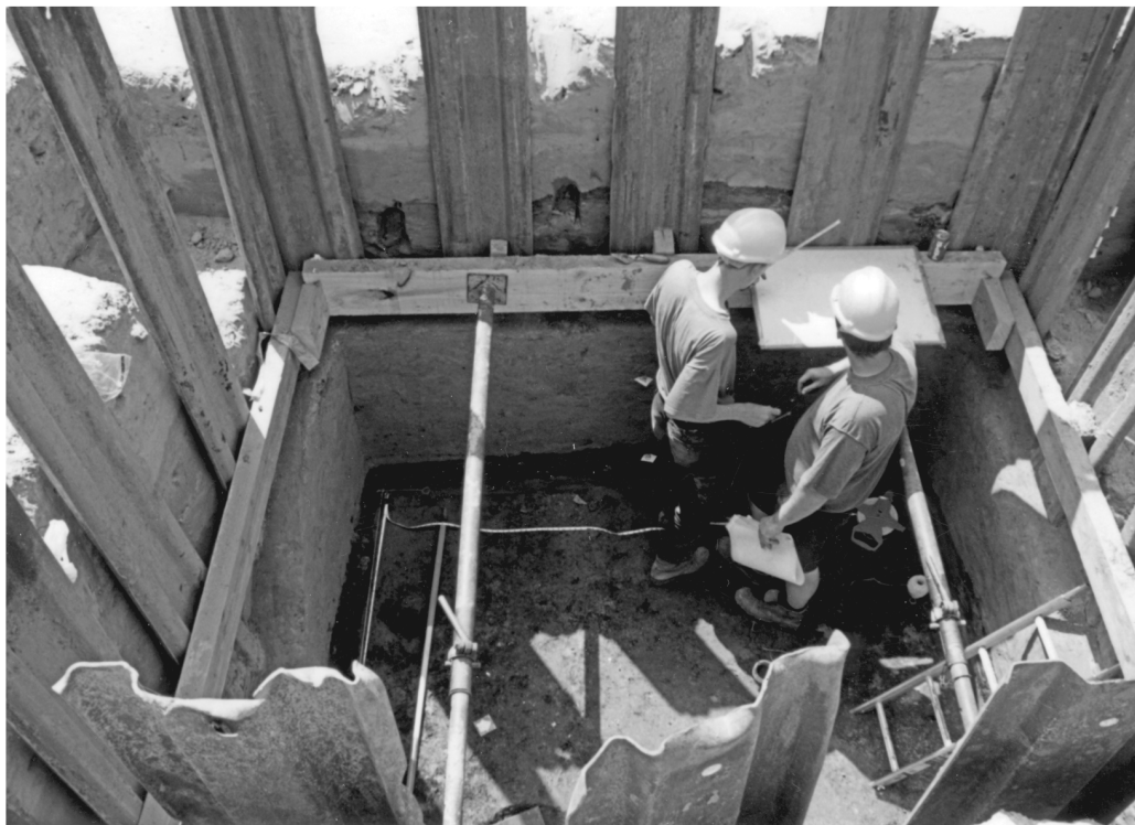
Plate 2 Working shots showing a) the excavation area (Area 1), looking east and b) one of the deeper trenches (Area 2), indicating the confined conditions
