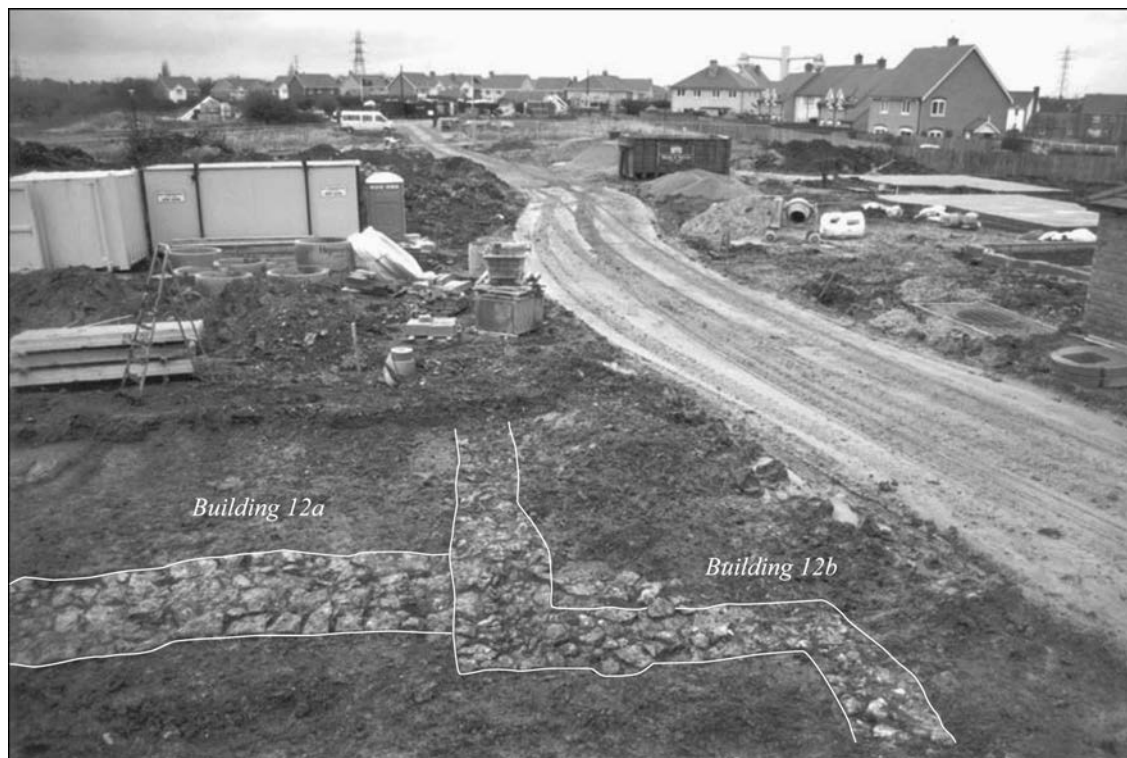
Plate X Building 12a and b (Area A), showing the impact of the development's haul road
