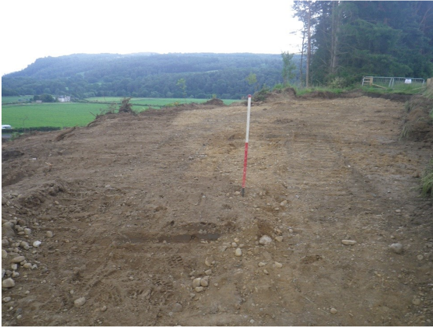
Plate 4. Ditch [212] prior to excavation, located on the edge of the steep terrace.
