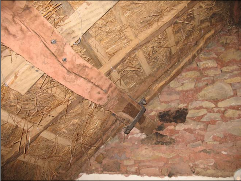
Figure 21: The east end of the northern purlin, after reinforcement, from the south-west.
