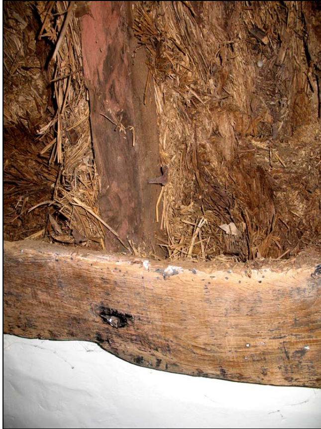
Figure 25: Detail of the south purlin showing a reused pegged rafter timber, with small pintle attached, from the north.
