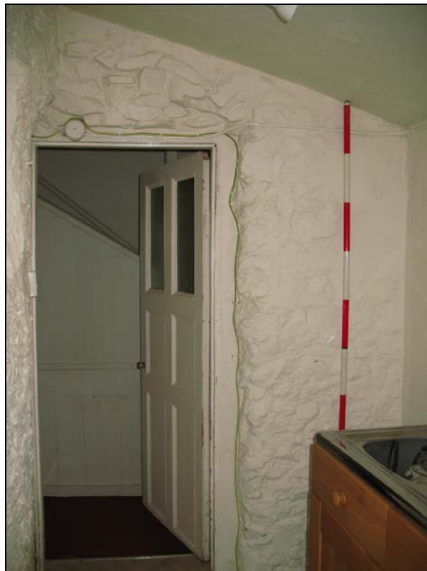
Figure 12: The west wall of the stair lobby, showing the disrupted wall fabric around the forced opening
