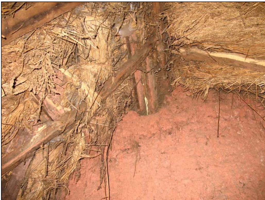
Figure 24: The reinforcing timbers at the west end of the ridge pole, from the east.
