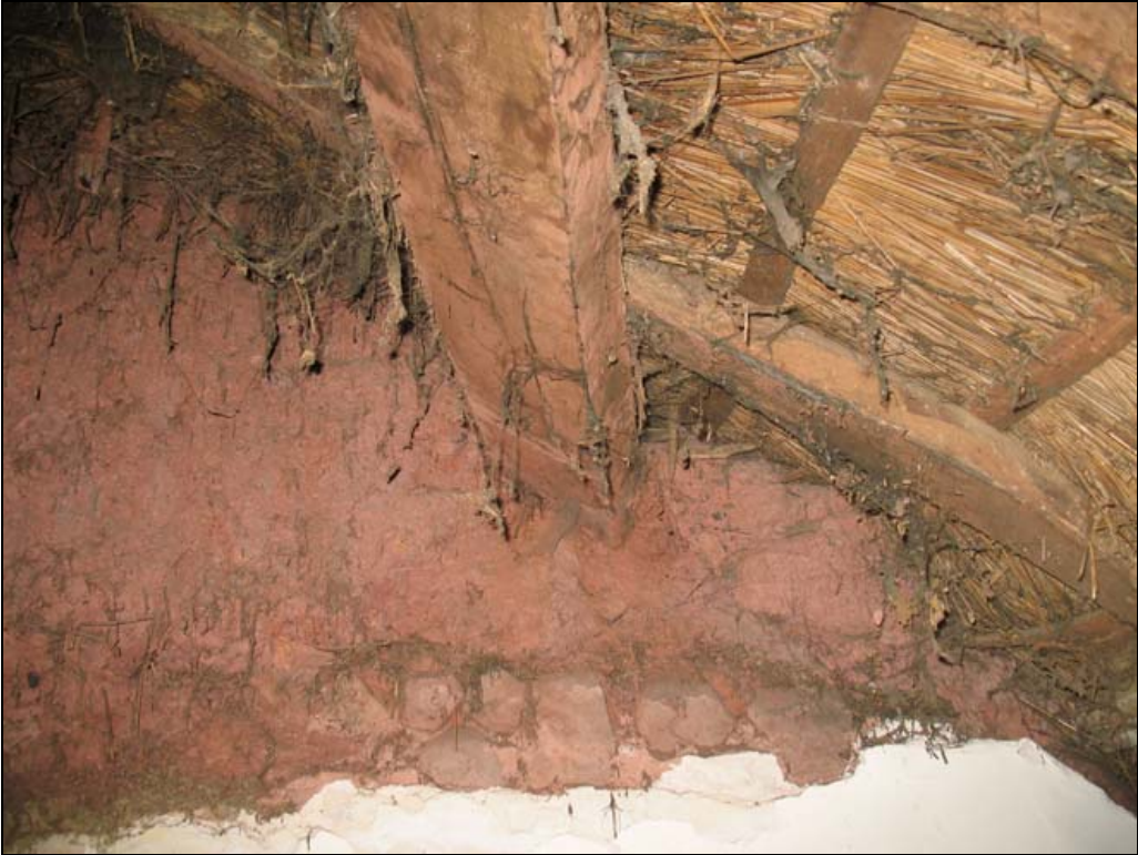
Figure 19: The western end of the north purlin, with stone packing below associated with the ceiling, from the east.
