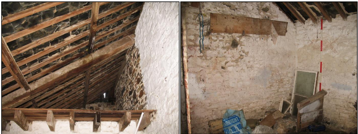
Figure 54: Left: Loft above Vestry accessed above north wall of Vestry, viewed from the south (2m scale).
