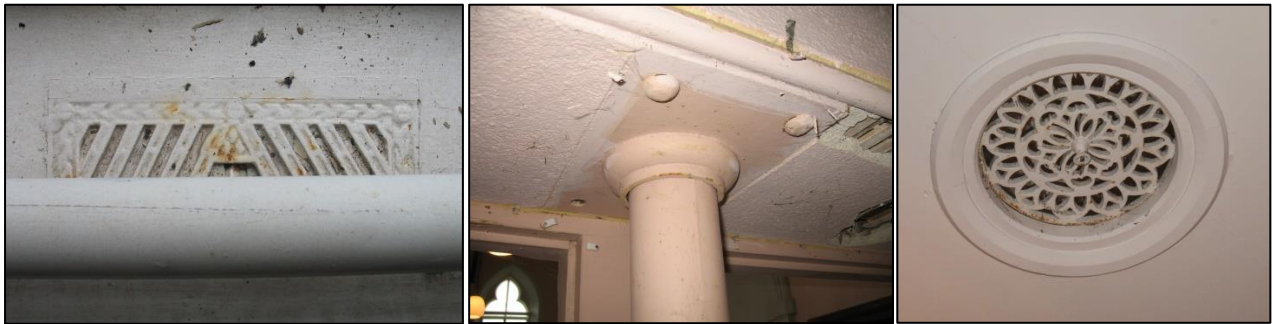
Figure 46: Left: Detail of vent example (partially obscured by modern pipe) in window sill in Hall. Figure 47: Centre: Detail of top of metal support in centre of opening between School Room and Hall, viewed from the northeast. Figure 48: Right: Detail of central circular vent in School Room ceiling.
