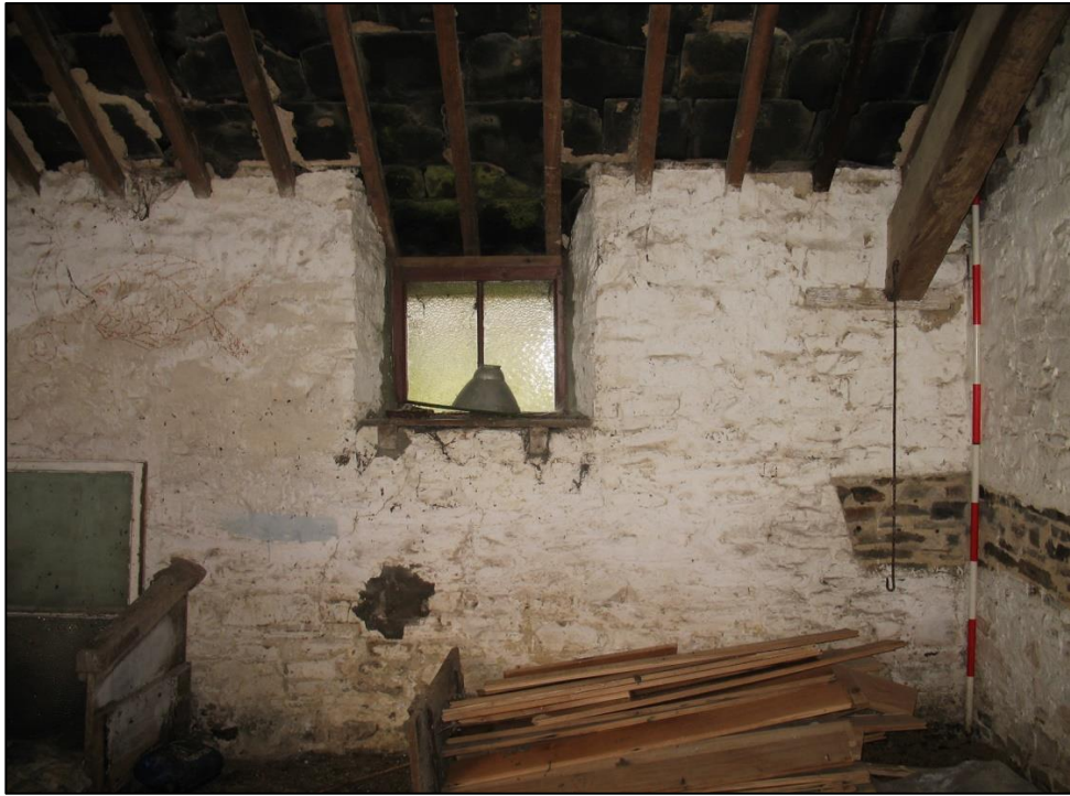
Figure 14: Interior west wall of Stable/Trap House, showing window opening and foot of principal rafter, viewed from the east (2m scale).
