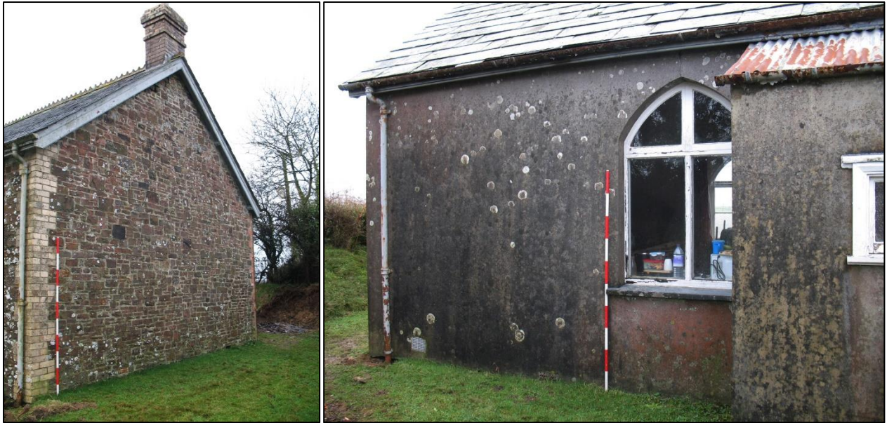
Figure 26: Left: North wall of School Room, viewed from the northeast (2m scale).
