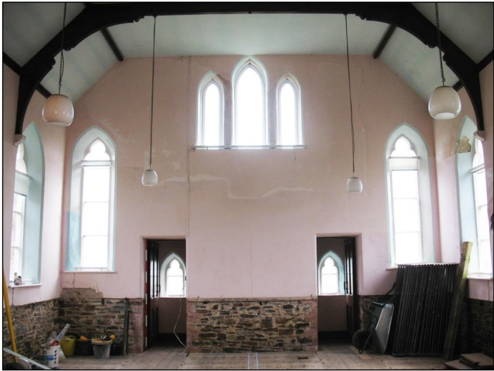
Figure 10: The Chapel Hall east wall, also showing ceiling with timber bracing below structural roof timbers, viewed from the west (2m scale).
