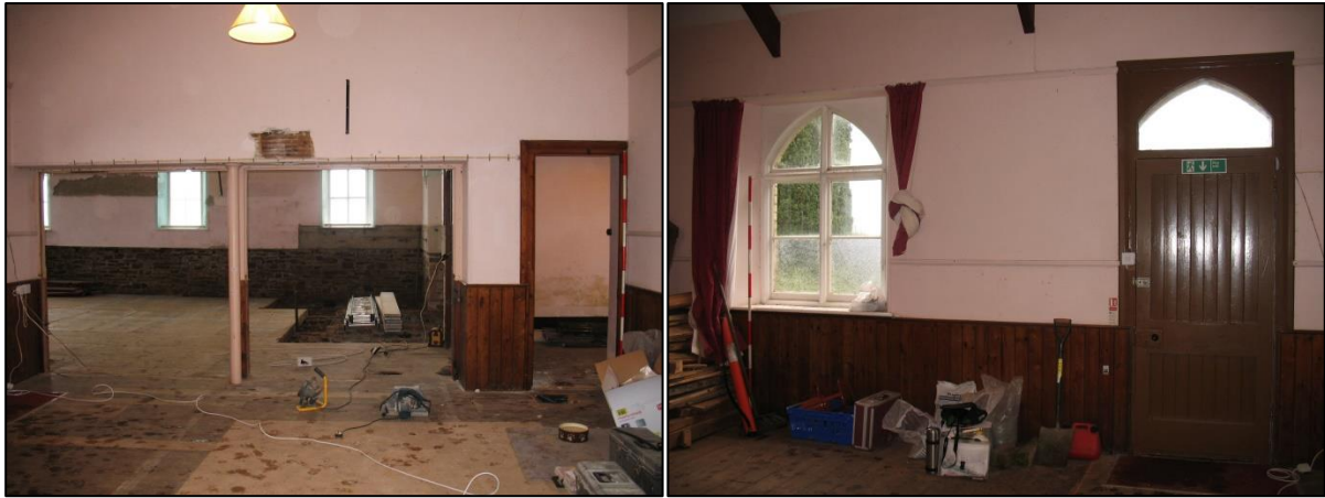
Figure 44: Left: School Room south wall, with openings into Hall and Vestry, viewed from the north (2m scale). Figure 45: Right: East wall of School Room, viewed from the west (2m scale).
