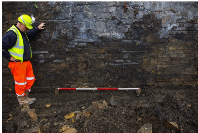
Figure 3.6 North-west facing showing above ground boundary wall and existing foundation trench after completion of grubbing works
