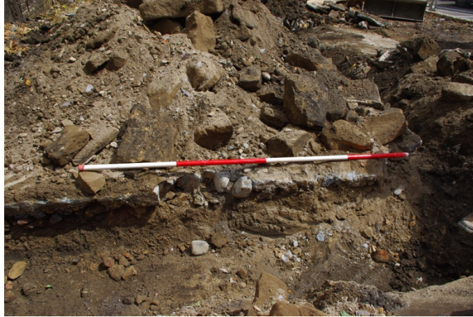
Figure 3.4 North-west facing showing existing south-eastern foundation trench after completion of the grubbing works
