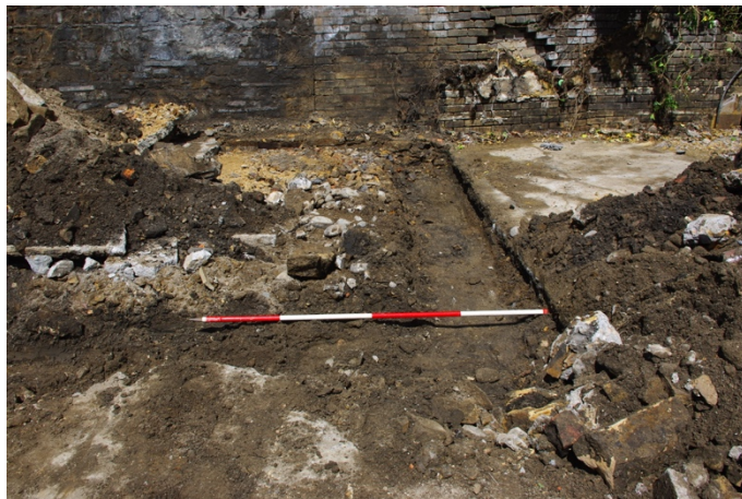
Figure 3.3 North-west facing showing three existing foundation trenches after completion of the grubbing works
