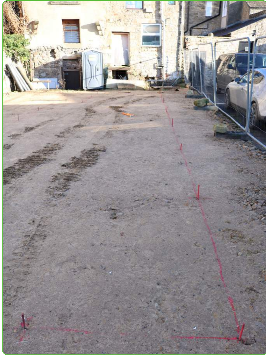
Detail showing the southeastern edge of the site with location of piles 24 and 25 in the foreground
