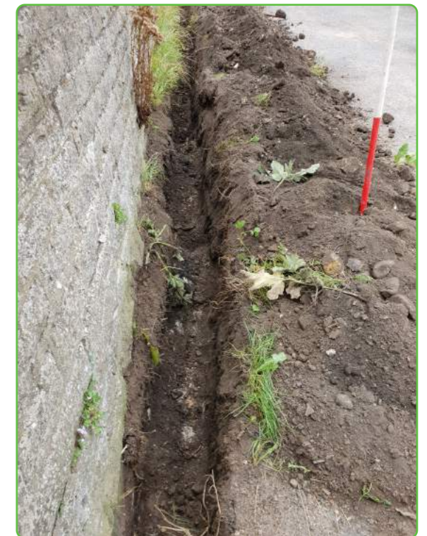
Detail of the cable trench running into the site from the northwest, facing southeast
