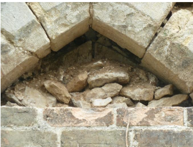
Fig 24: Bay 10, with upper brickwork removed, showing rubble core and back of tracery behind
