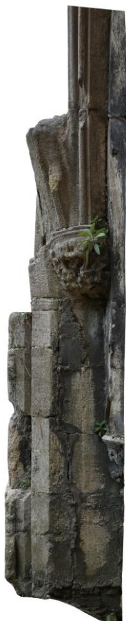
Fig 20: Wall stub north of doorway, on west side of wall 17; rectified. Note the window jamb, vault corbel and vault ribs (The Downland Partnership)
