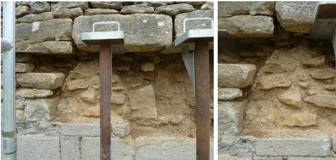
Fig 10: Third lancet from north, showing mortars behind facing. The pale lime-based mortar of the lancet is clearly visible against the darker, clay-based mortar of the re-facing.
