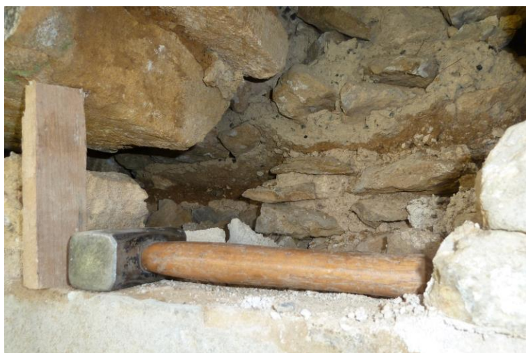
Fig 21: Above bay 10, showing tilted horizontal building break; mortar samples taken both sides of break
