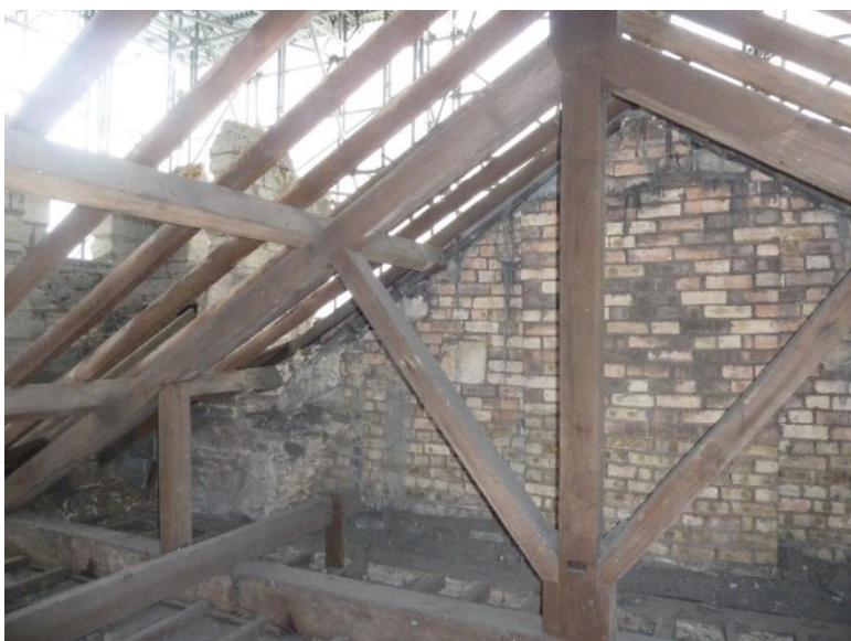
Plate 42 (Archive image PCKC 631) Knights' Chamber roof space, view of north gable with new brickwork Photograph: Jackie Hall
