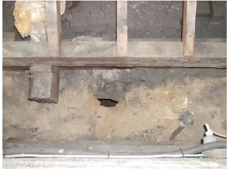
Plate 71 (Archive image: PCKC 133) Bishop's Gate roof east side: showing the location of the flue. Photograph: Caroline Atkins
