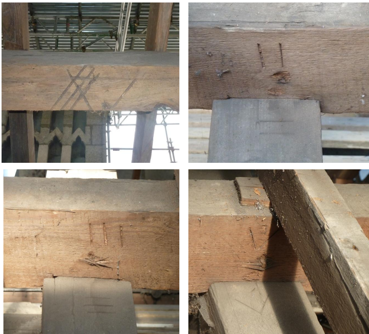
Plate 39 (Archive image PCKC 637, 645, 646, 648) Knights' Chamber roof: selection of carpenter's marks on trusses Photographs: Jackie Hall
