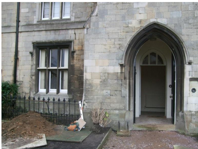
Plate 55 (Archive image PCKC 029) Trial Pit 2: location to the east of the porch. Photograph: Caroline Atkins
