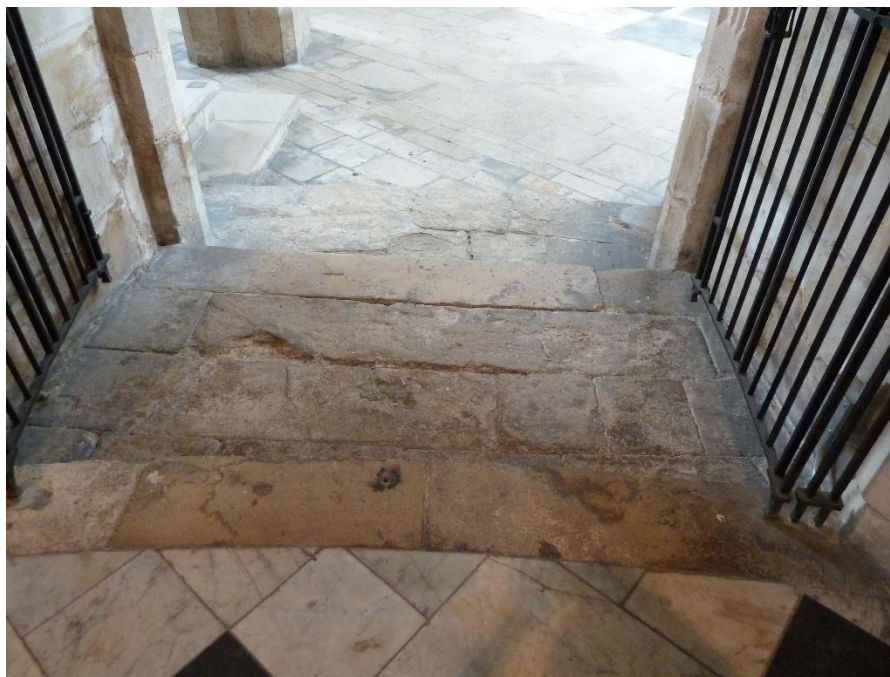
Plate 2 View of ramp location from top showing worn middle and lower steps. Photograph: Jackie Hall (2011)
