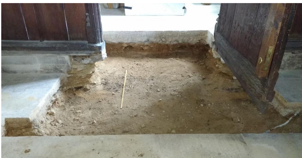
Plate 12 (Archive image PCTAR 40) Whole of trench, viewed from treasury Photograph: Jackie Hall
