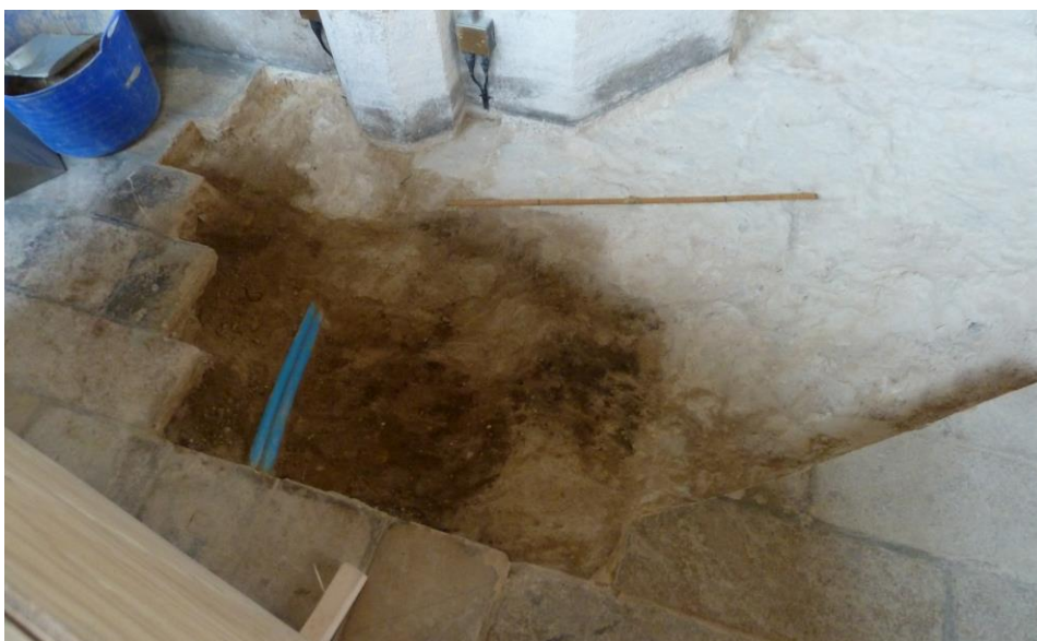
Plate 10 (Archive image PCTAR 52) West end of trench, showing concrete, burial earth and pipes Photograph: Jackie Hall
