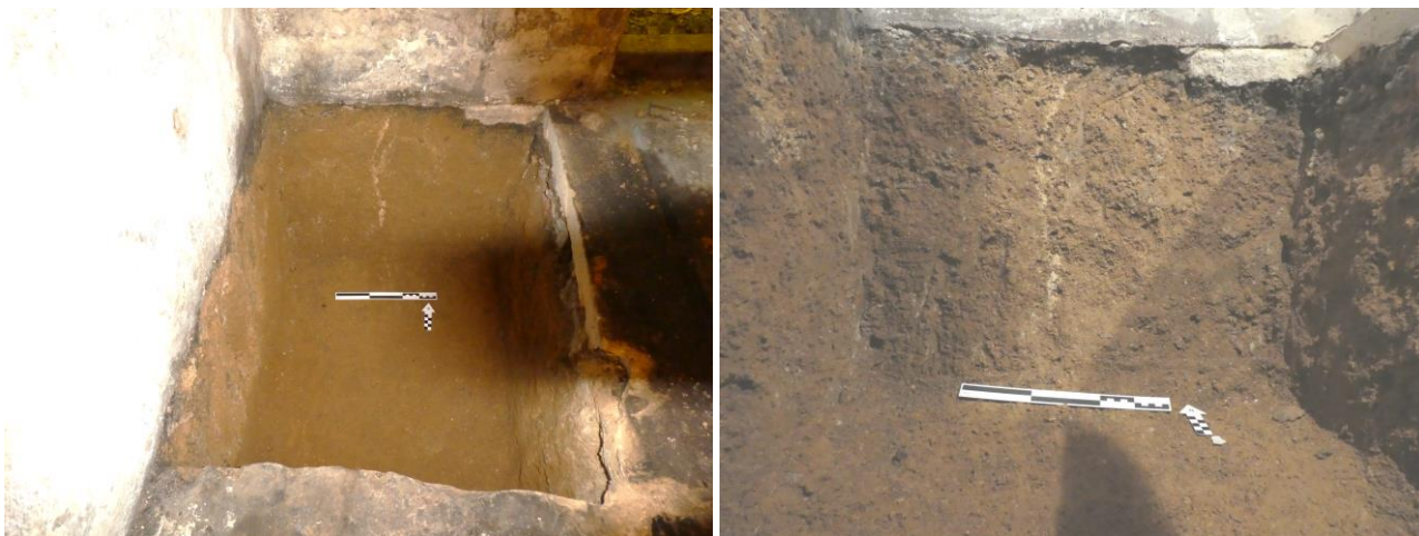
Figure 15: Pit for boiler room sump pump: (left) general view, looking north; (right) north section, showing solid sand and gravel (scale = 0.30m)
