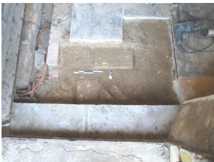
Figure 6: Area excavated for new duct in north aisle, immediately in front of step to north door, looking south (scale = 0.30m)
