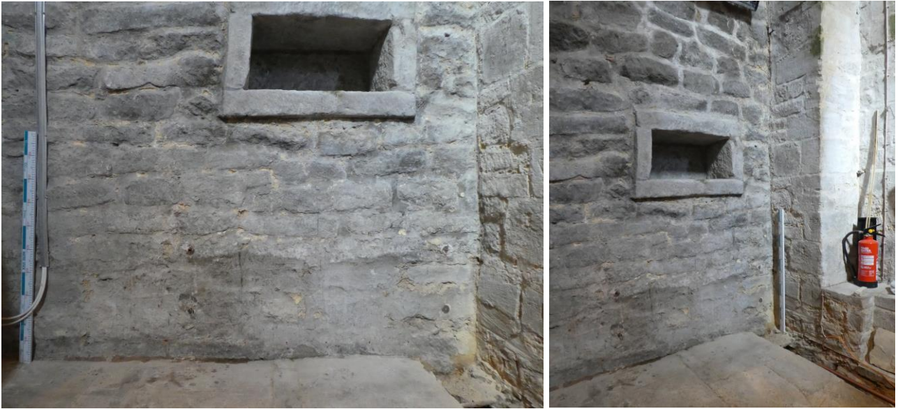
Figure 16: North wall of tower, temporarily exposed; 13th-century insertion at right hand side (scale = 1m)
