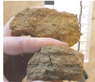
Figure 12: The mortar floors: (upper) the upper floor; (lower) the lower surface. Both samples disintegrated after they were photographed
