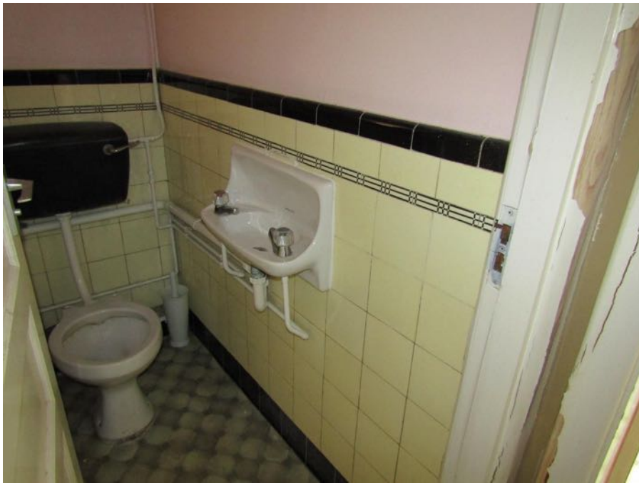
Figure 23 - delicate detail in WC
