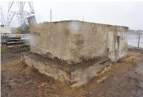
Photo 4.1: Western and southern elevation of the pillbox. Showing step around open chamber.
