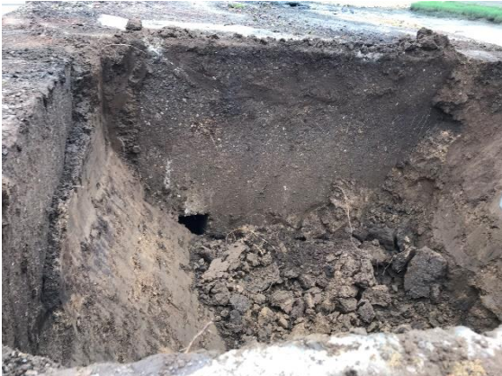
Photo 4.5: Top of open chamber, with infill partially removed. Top of doorway to roofed chamber partly shown.
