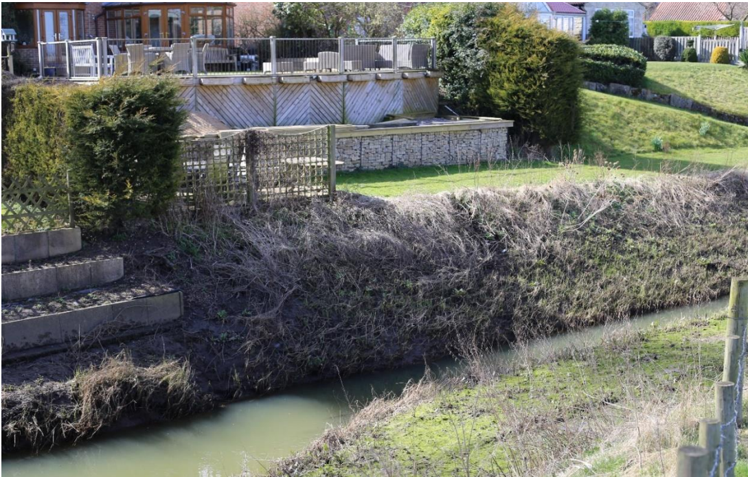
Photo 3: Part of Ulleskelf flood barrier
