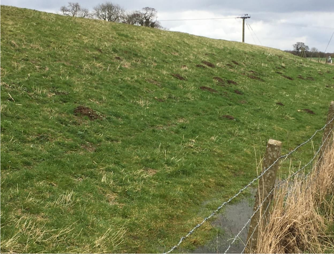
Photo 2: Close-up View Bowlam Bank illustrating uneven nature
