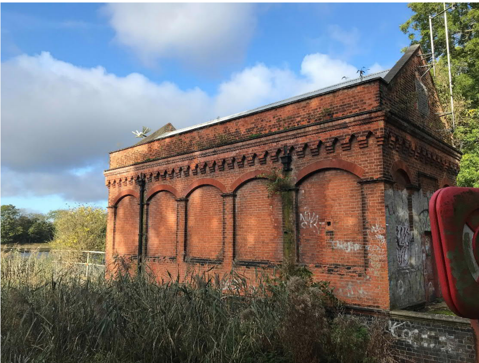
Figure 4.5: Pump house at the eastern edge of Hampton Distribution Reservoir, facing north
