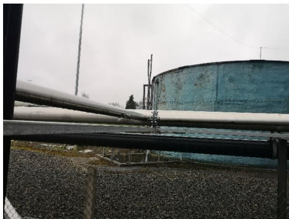
Figure 7 Existing DN150 CHP Biogas pipework to be removed
