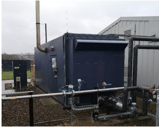
Figure 8 Existing containerised CHP with exhaust stack and air intake vent which will be removed. Hot water pipes to top right elevation will be redirected to the new CHP area via a new pipe bridge.
