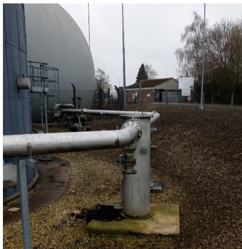
Figure 11 Existing condensate pot to be replaced.
