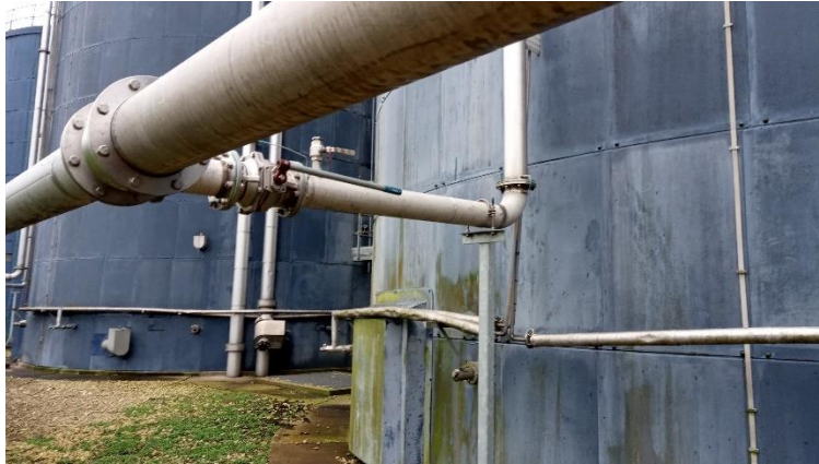
Figure 10 DN150 Digester outlet pipework where condensate pots are proposed for installation.
