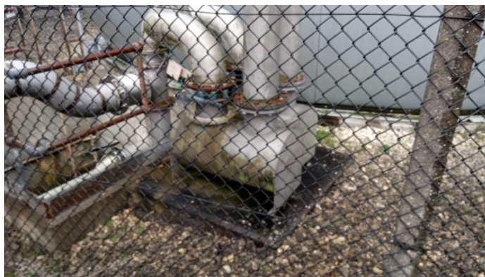
Figure 12 Existing P/VRV to be removed on Gas Holder feed pipework.
