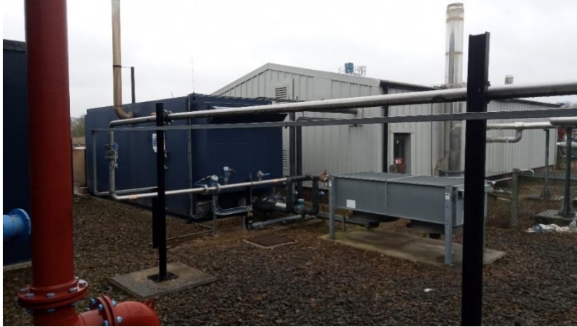
Figure 13 Existing CHP Plant
