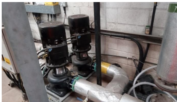
Figure 9 Existing water recirculation pumps to be replaced
