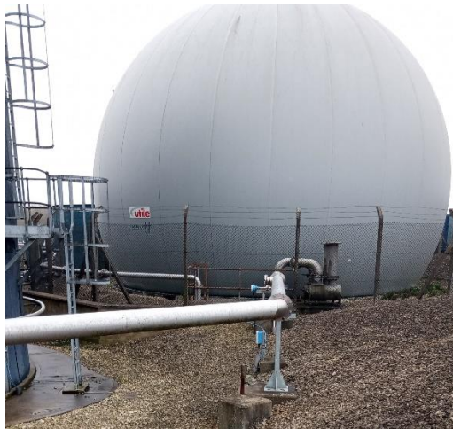
Figure 6 Pre Gas Holder Pipework where 1No. new Tee piece CHP biogas feed will be installed
