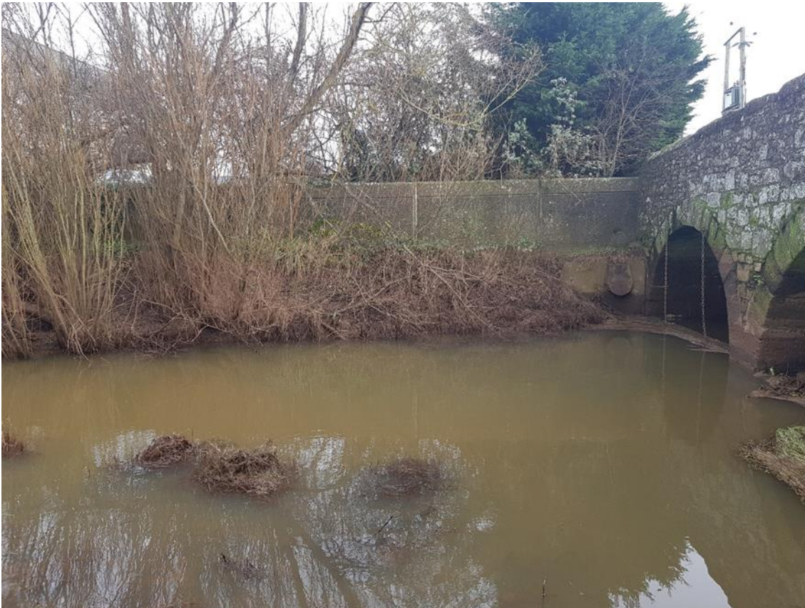
Figure 2: Existing concrete flood defence wall, north of Clyst St Mary Bridge, looking east
