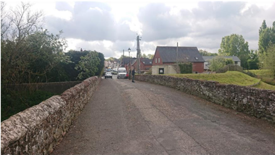
Figure 2: The eastern extent of the Clyst St Mary Bridge showing modern concrete flood wall and embankment, looking east.
