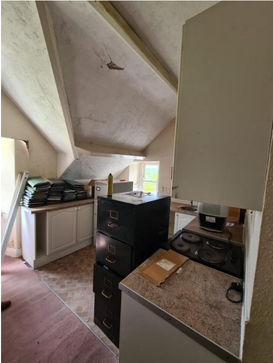
Figure 4.13: Former second floor flat kitchen in the south-western corner of the Original School Building.
