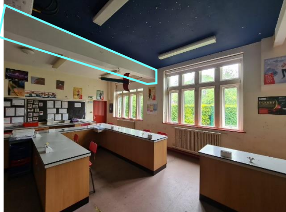
Figure 5.54: Eastern classroom in the 1935-7 Science Building with downstand beam highlighted in blue
