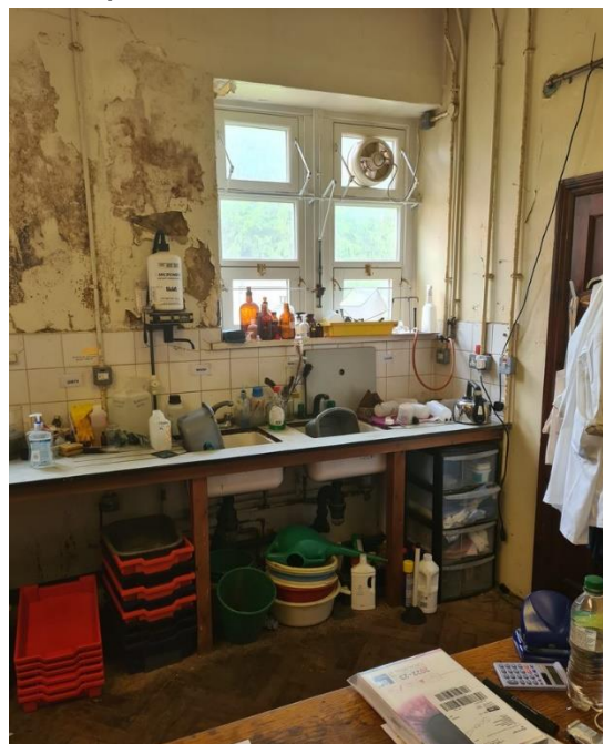
Figure 5.51: Store cupboard, showing areas of damp
