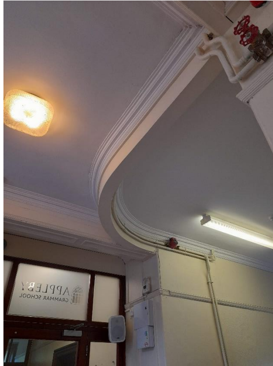
Figure 4.29: Downstand beam from the former partition between school and flats within the Original School Building
