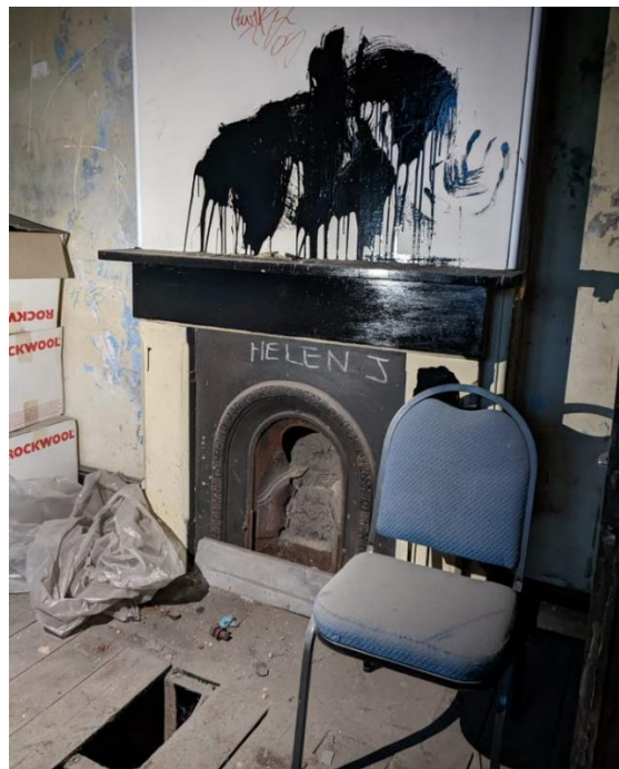
Figure 5.126: Fireplace and graffiti on the third floor (EFAA).
