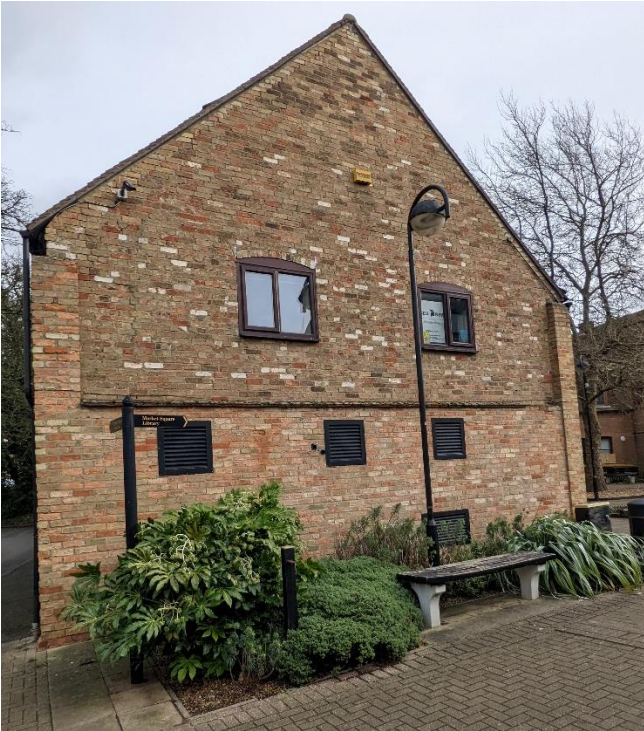
Figure 4.12: Building to the east of proposed development area 3, with evidence of alterations to original historic structure
